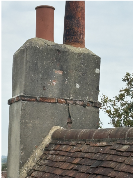
3. 8 South Street: Rear chimney, render in poor condition to be replaced
