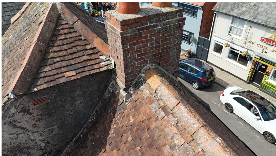
2. 8 South Street: Front chimney (southern) failed/ineffective weathering to be replaced
