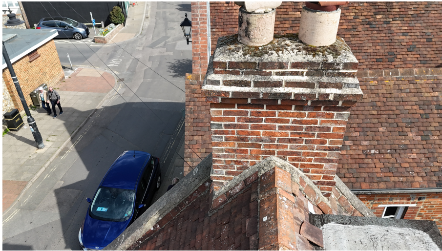
1. 8 South Street: Front chimney (northern) failed/ineffective weathering to be replaced
