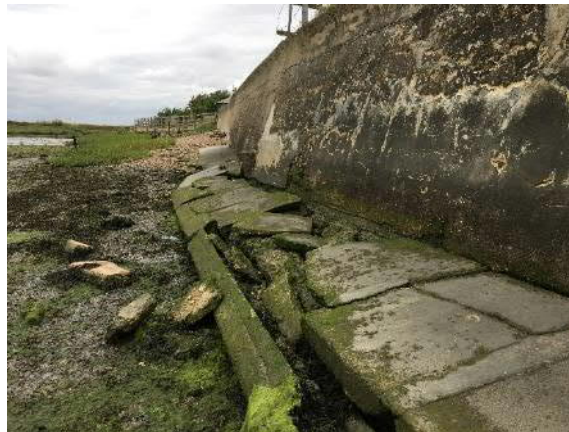
Figure 4-3: Structure 2 sub-unit ODU1b East – failed apron
