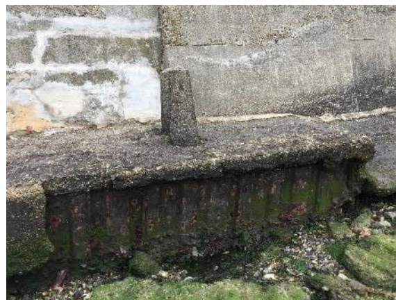
Figure 4-4: Structure 2 sub-unit ODU1b – exposed steel piles
