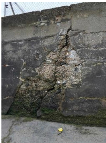
Figure 4-5: Structure 2 sub-unit ODU1b – vertical crack in seawall
