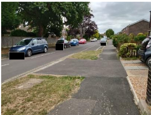
Photograph 21: Brights Lane Footway Conditions
