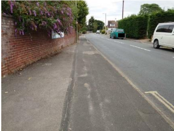
Photograph 25: Manors Road footway conditions
