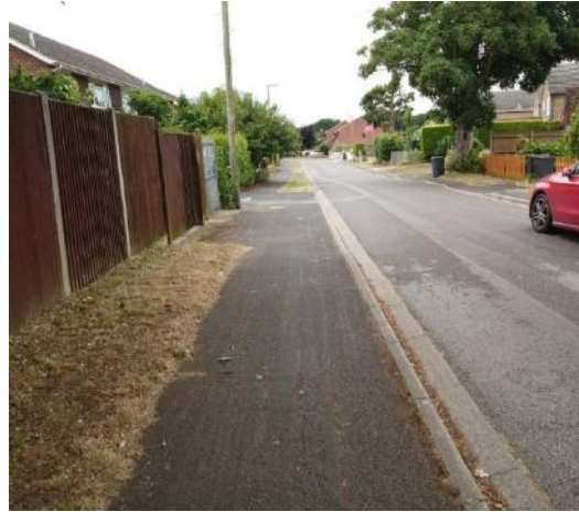
Photograph 2: Saltmarsh Lane Footway Conditions
