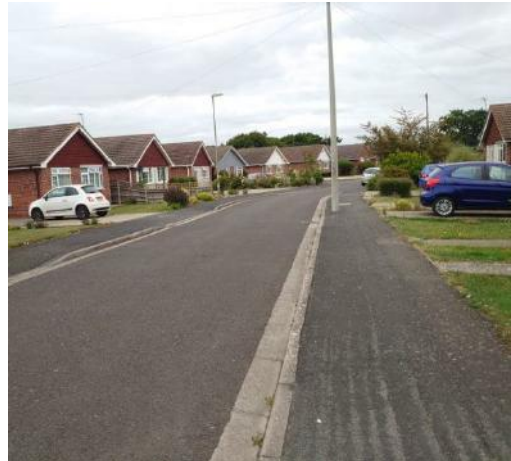
Photograph 4: Denhill Close footway conditions
