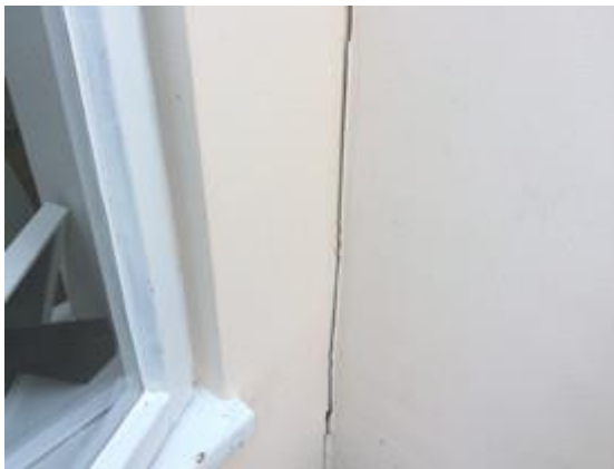
Picture 3: Internal cracking to conservatory
