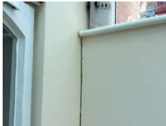
Picture 2: Internal cracking to conservatory
