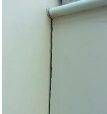
Picture 4: Internal cracking to conservatory
