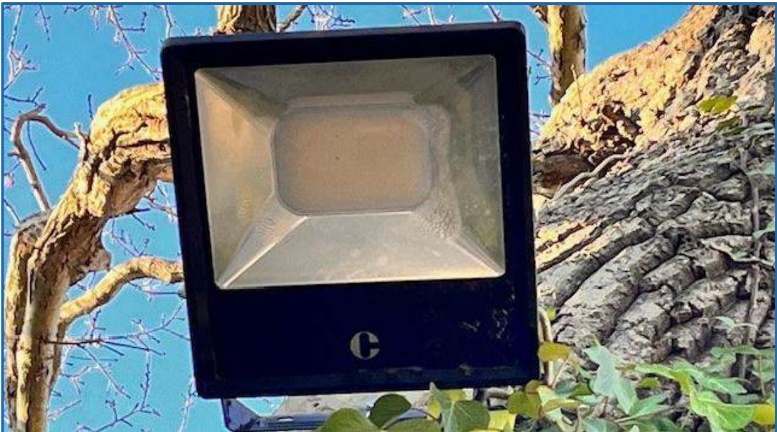
Figure 18: Close up Picture from Underneath Light Number 2 from Figure 16 and Figure 17
