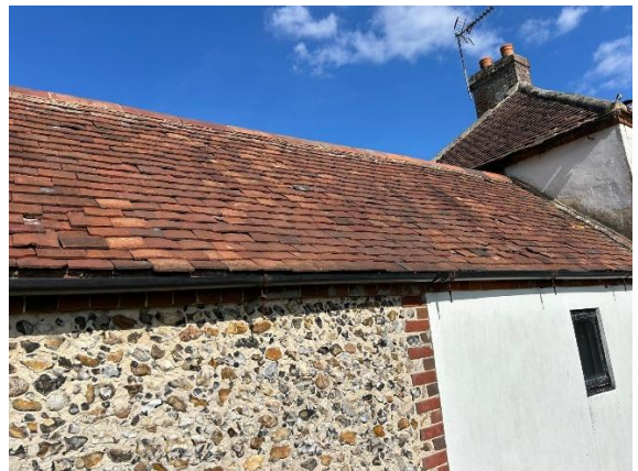
Image 8. A close-up of the single-storey extension showing gaps in the roof tiles.
