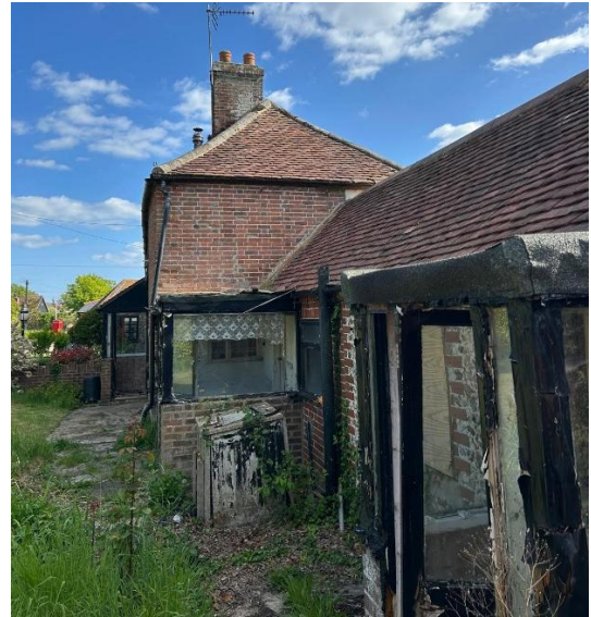
Image 6. The eastern elevation of the building viewed from the north, looking south. Shows gaps in roof tiles and a missing ridge tile.
