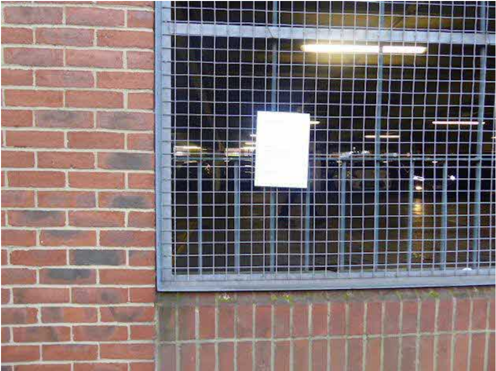
Photograph 8 – Further view of the notice on the north elevation.
