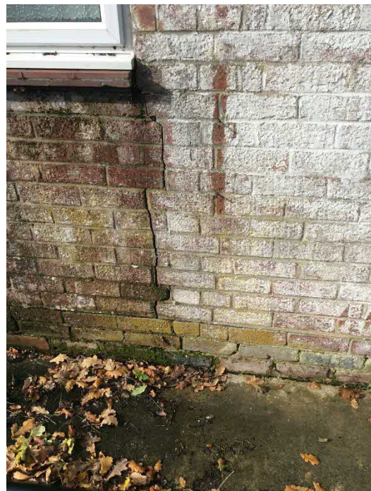
Crack to rear wall
