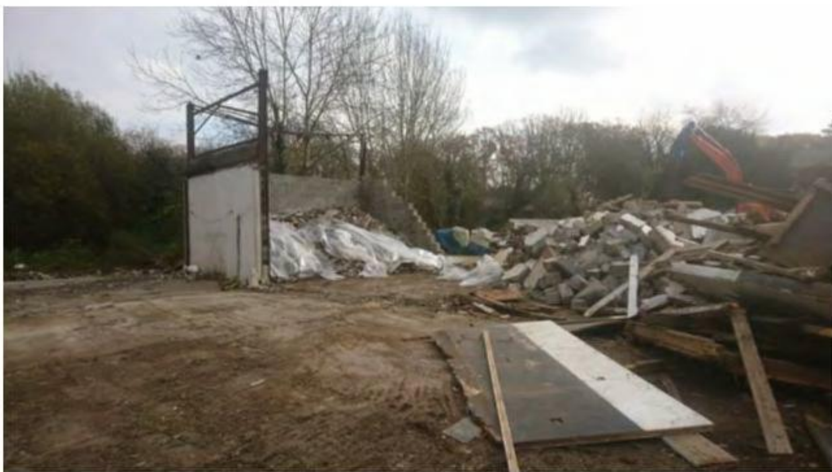
Plate 2 View of demolished former stables, with stockpiled wastes and possible ACM materials
