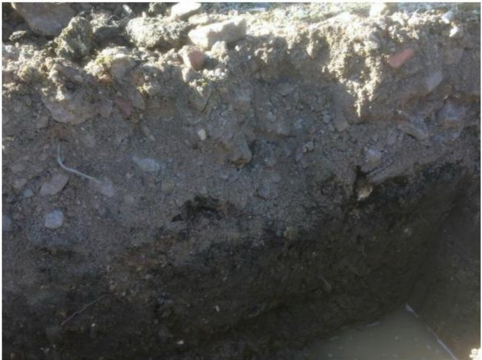
PLATE 6 – TP2A relocated but groundwater was still at 1.1m possibly in made ground so abandoned
