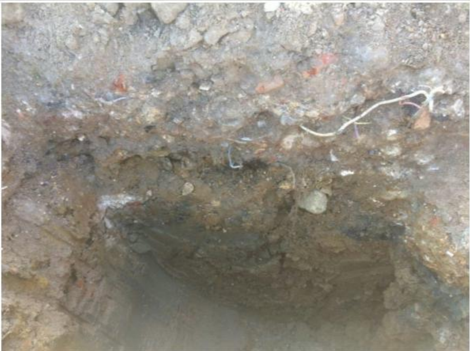
PLATE 8 – TP2B abandoned due to high, possibly due to water running along old pipe gravel surround
