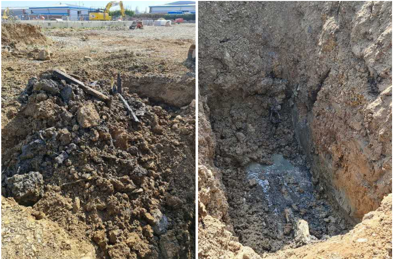
Figure 21 – Typical visual evidence hydrocarbon contamination (staining and odour).
