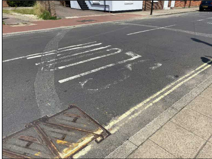
Photograph 2: Double Yellow Lines along Queen Street
