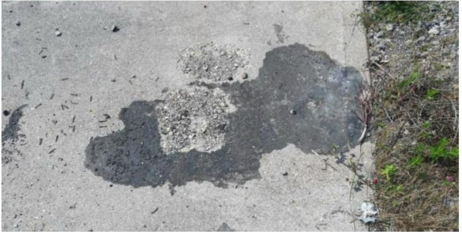
Plate 21 13c - Dark staining (no odour) to concrete slab.
