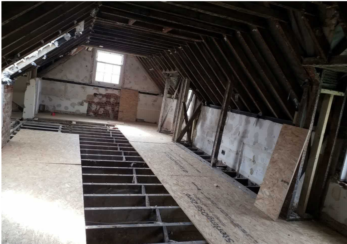
Photo 14 (Roof showing alterations)
