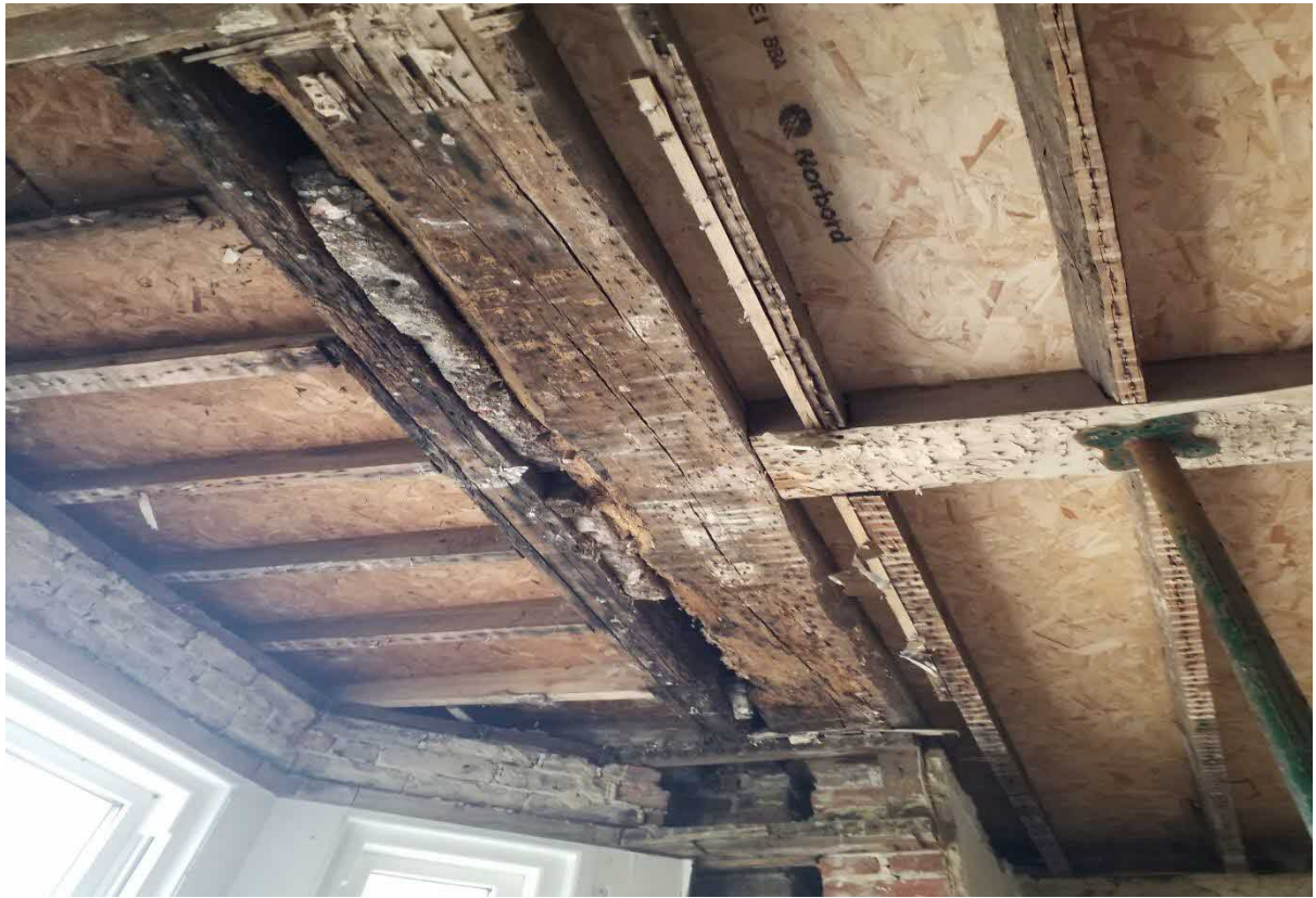
Photo 9 (Timber beam lack of connections)
