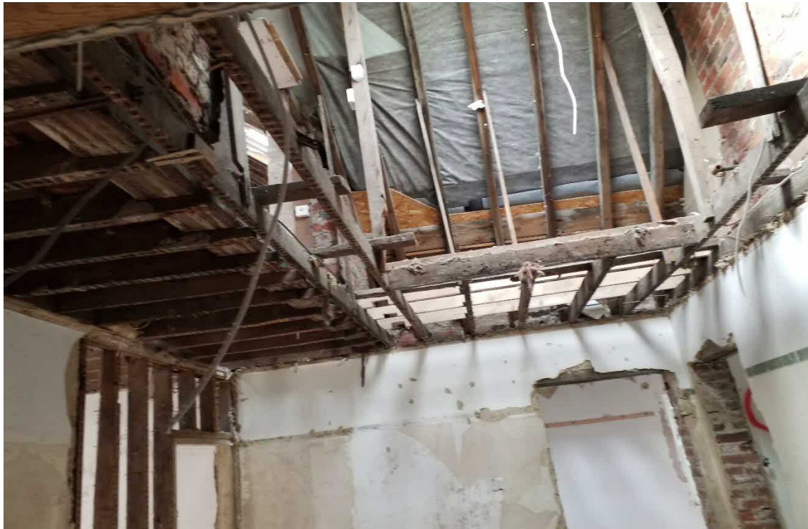
Photo 22 (Poor support to both roof and floor opening)
