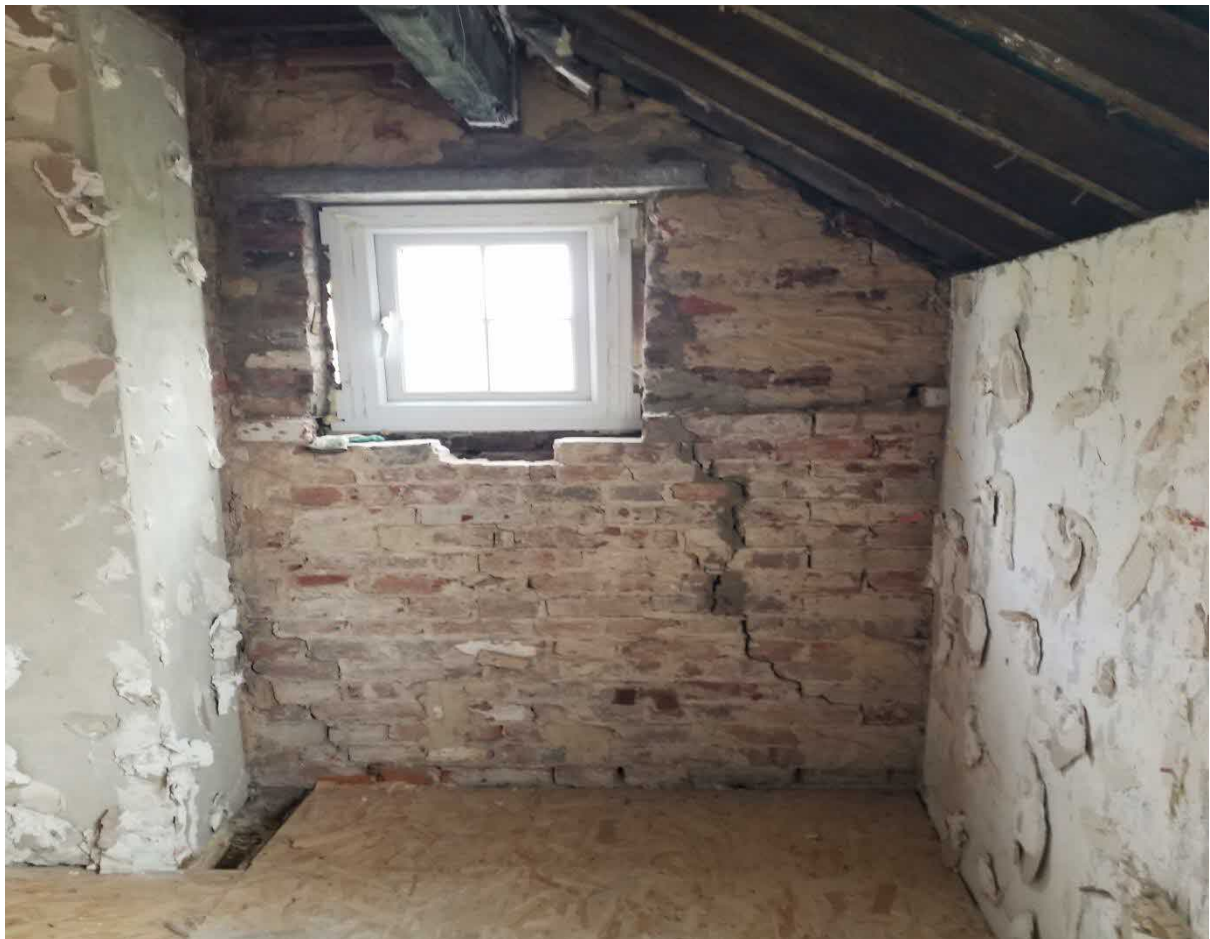
Photo 21 (Cracking to side gable internal – Concrete lintel)
