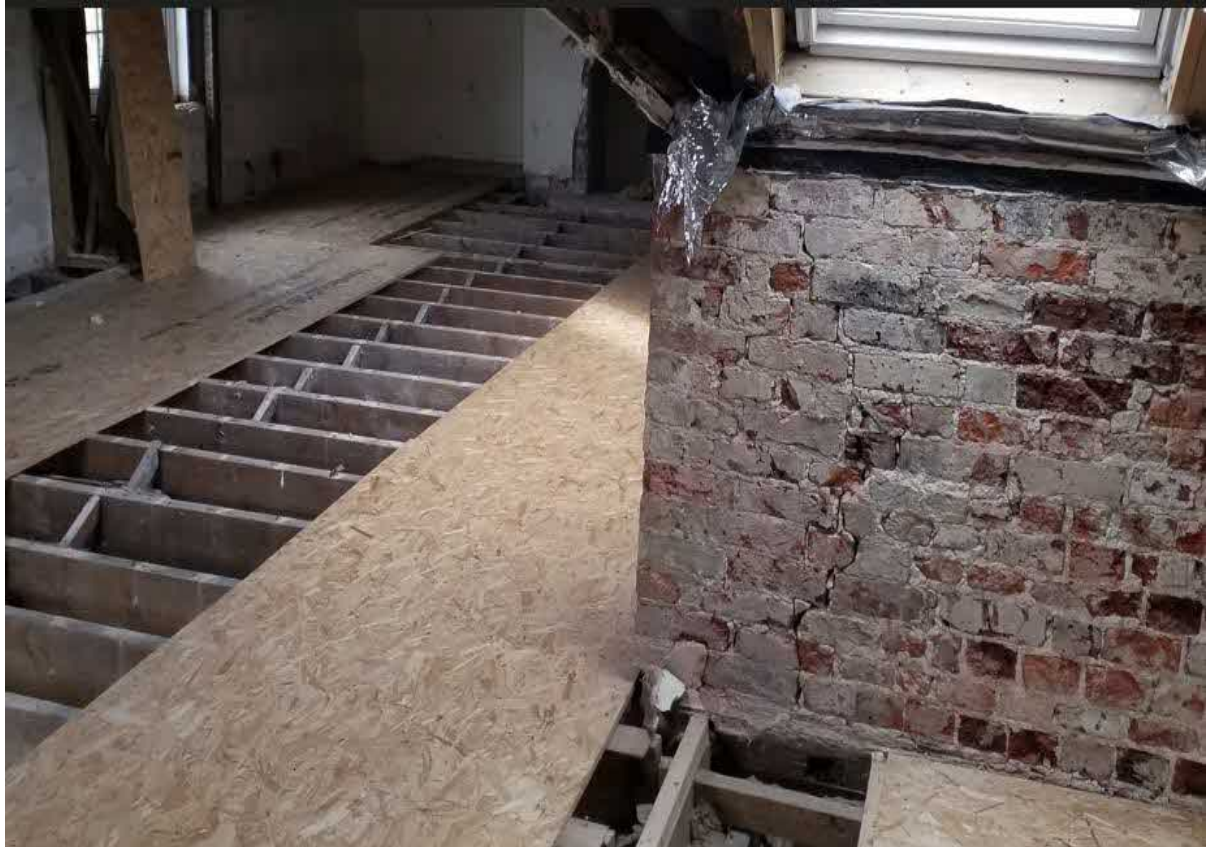
Photo 7 (Roof supporting wall cracking)
