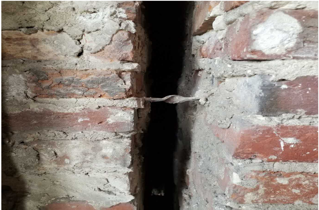
Photo 6 (Wall tie design found)
