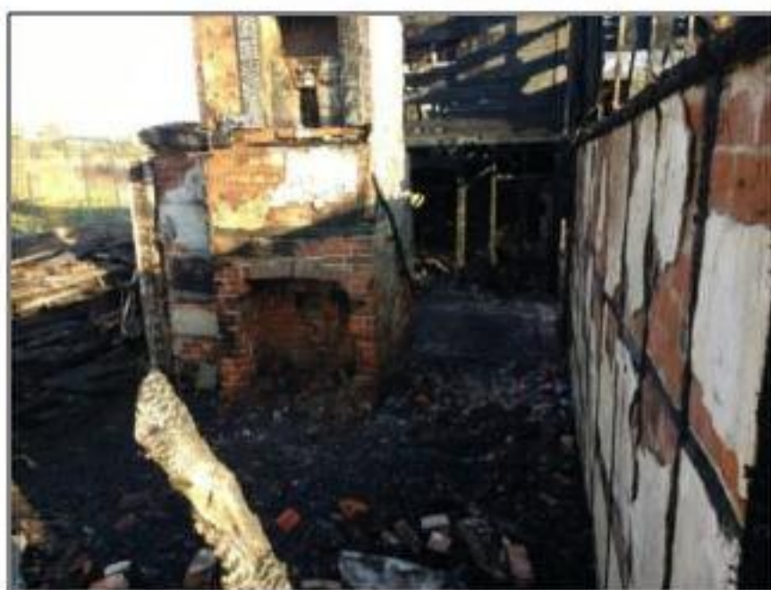
Figure 24: The cottages after the devastating fire (Jan, 2019)
