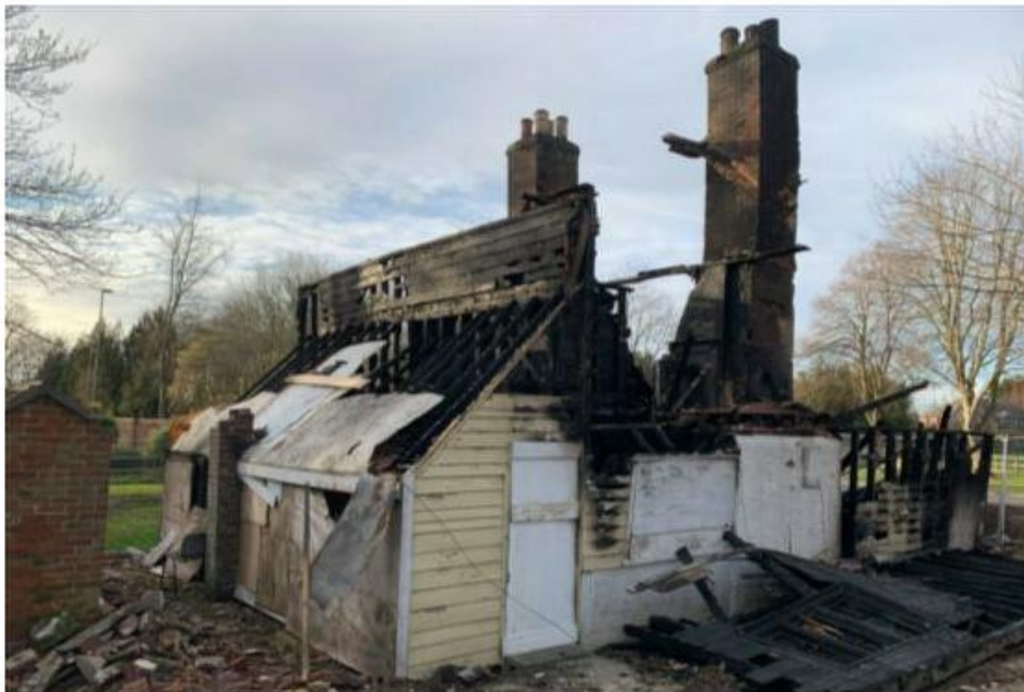
Figure 3: Post-Fire Damage (Jan 2019)
