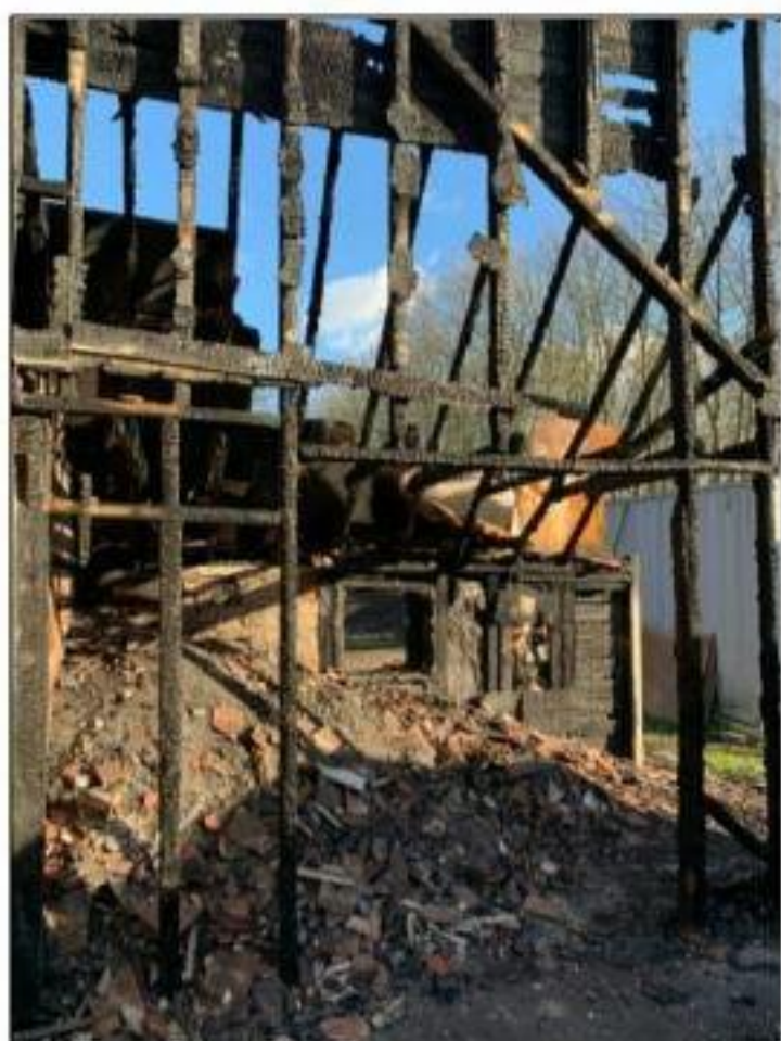
Figure 23: The cottages after the devastating fire (Jan, 2019)
