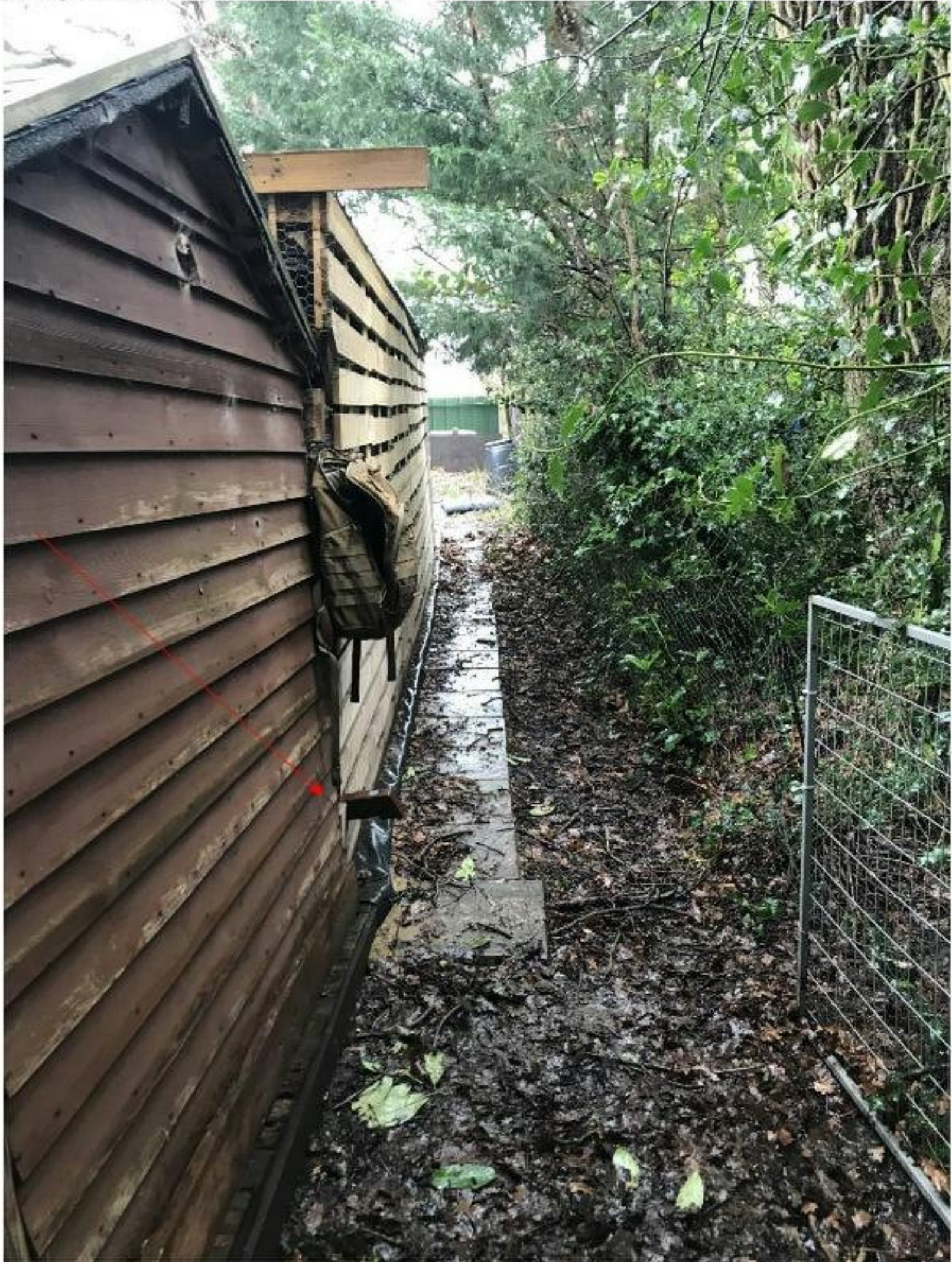
Photo 3. Rainwater outlet marked with an arrow
