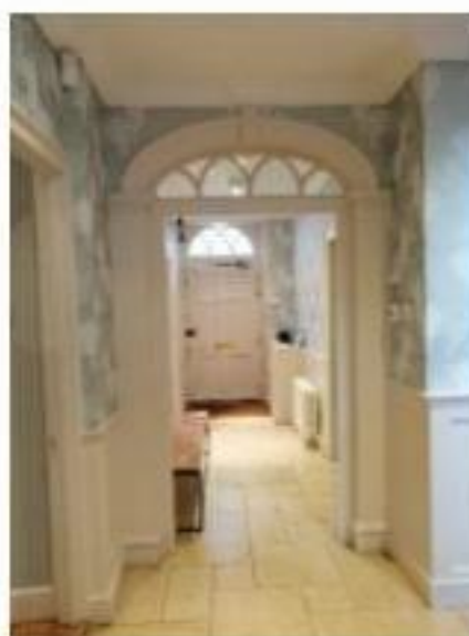
Existing entrance flooring to be replaced
