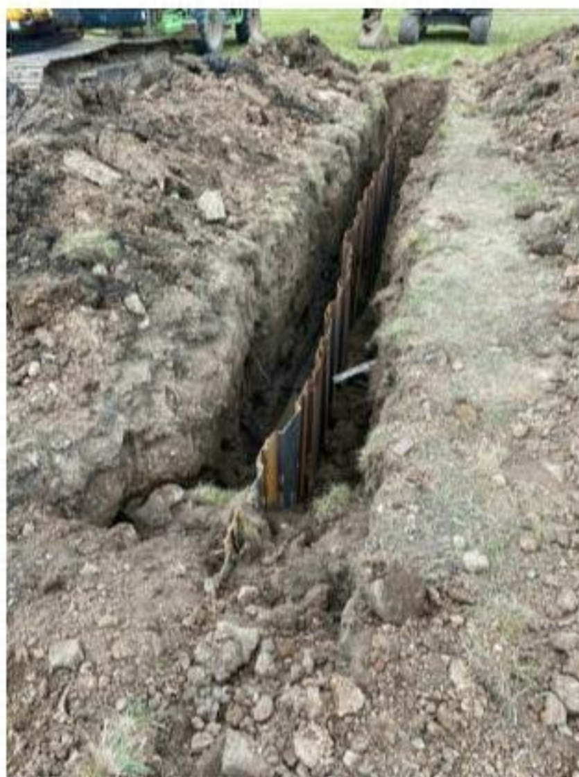
Photo 7: Landward return at end of contamination migration barrier (Photograph provided by Yachthaven).
