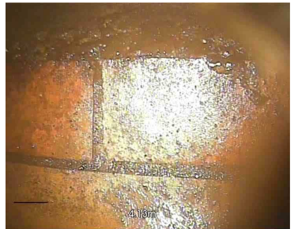
2, 00:00:23, 4.13 m Finish node, manhole, reference: SU720610KD, Buried
