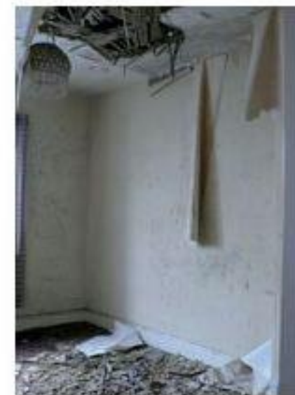
Room on eastern boundary - water damaged ceiling
