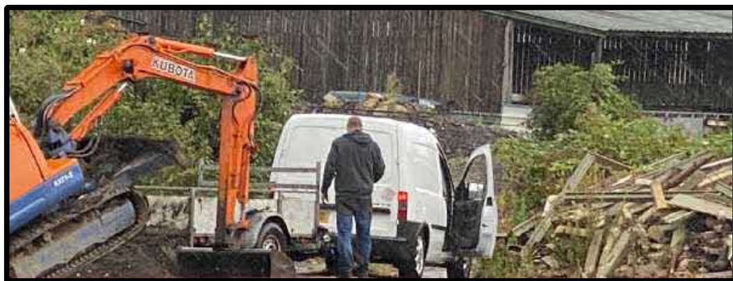
Third party business Phillips Fencing and Landscapes depositing waste earth at the tip site, without transfer notes or other permits. Not agricultural use. Photograph date 25/07/2020
