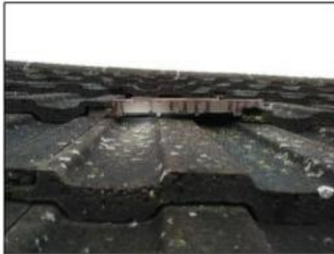
Figure 6: Gap under vent
