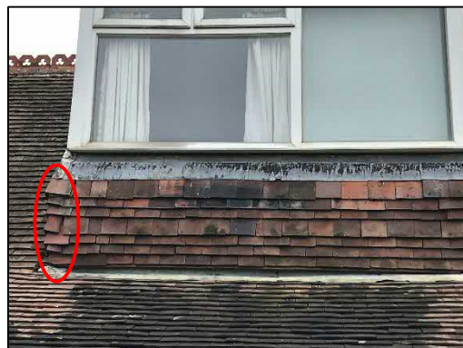
Figure 8: Lifted tiles around dormer window
