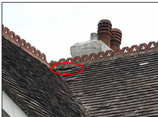
Figure 7: Missing tiles along roof ridgeline
