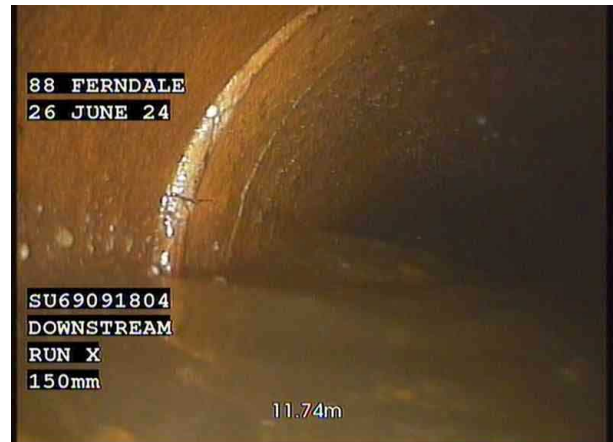
2, 00:01:12, 11.74 m Crack, circumferential at joint from 9 o'clock to 11 o'clock
