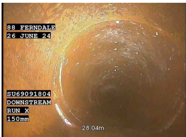
3, 00:02:39, 28.04 m Crack, circumferential at joint from 6 o'clock to 10 o'clock
