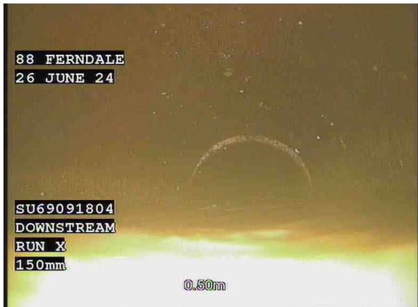
1, 00:00:11, 0.50 m Settled deposits, other, 25% cross-sectional area loss, start, Debris
