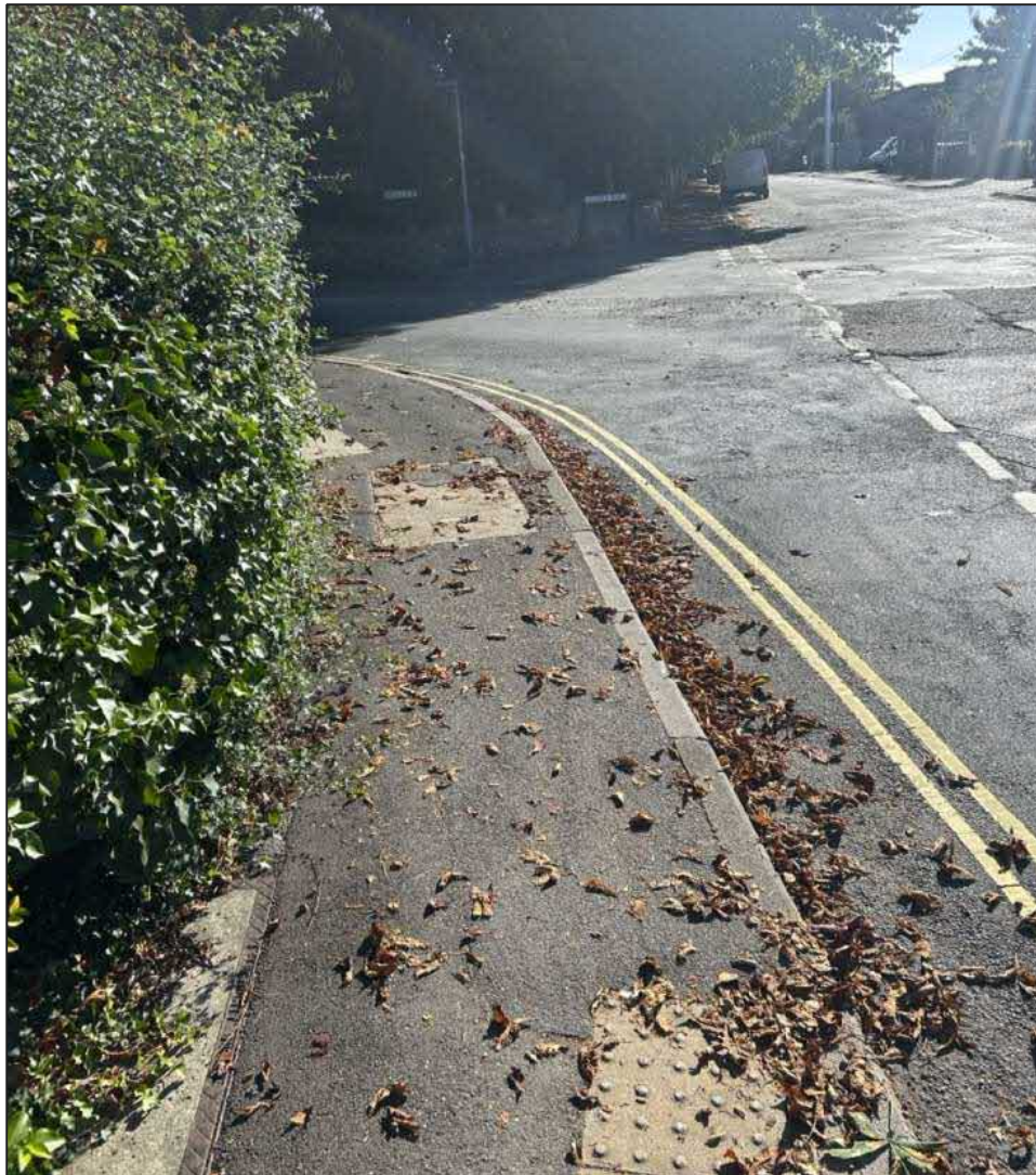
Photo 1: Lack of Visibility at the New Lane / Eastern Road Intersection
