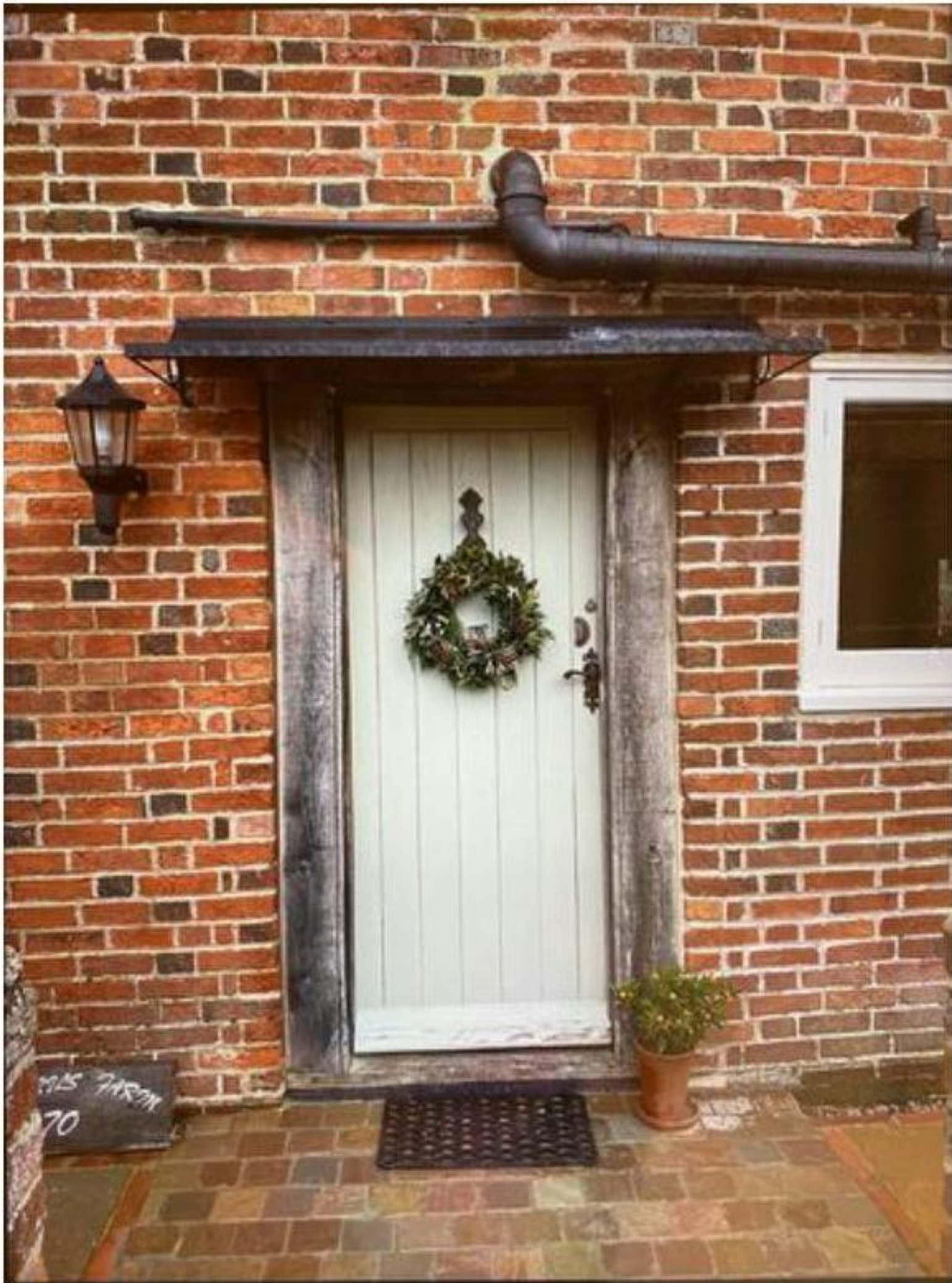
Image 8 – the existing kitchen door is subject to direct weather penetration
