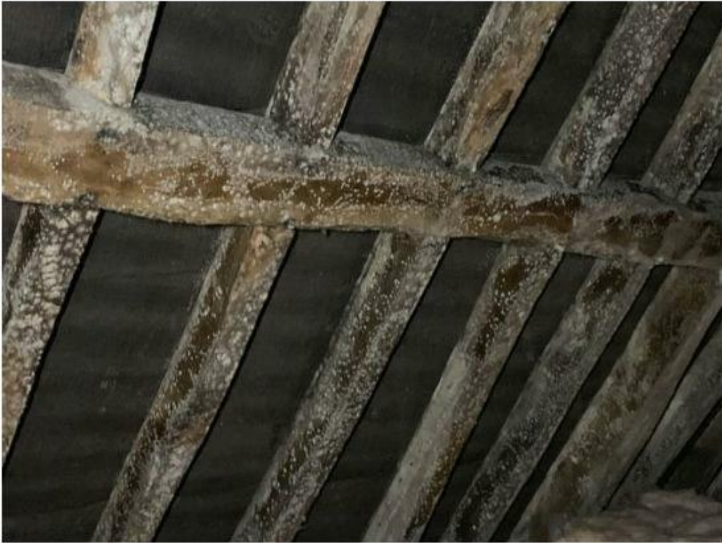
Image 2 – severe condensation within the roof space
