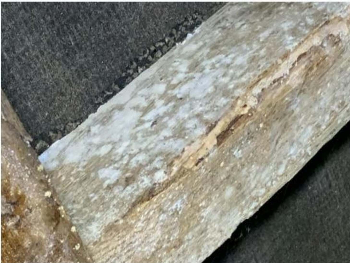
Image 3 – close-up of the severe condensation resulting from the moisture in the roof
