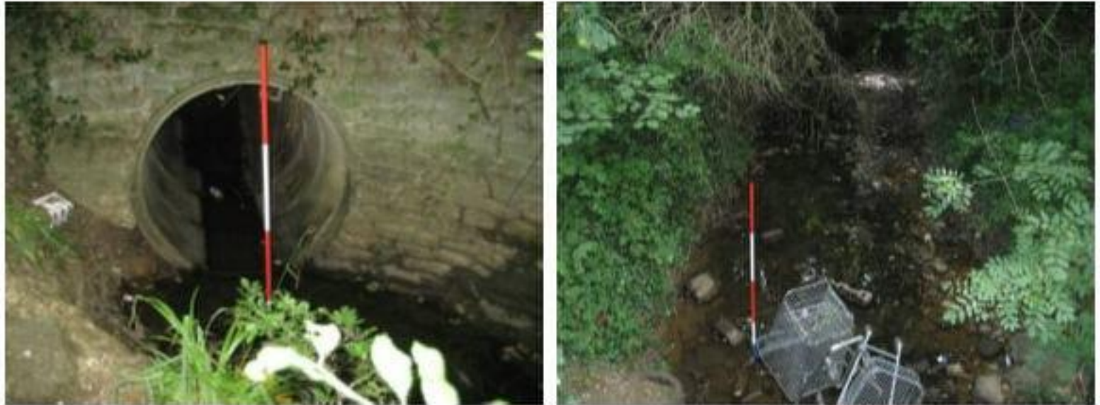
Photo 1: Major culvert & dumping in Riders Lane
