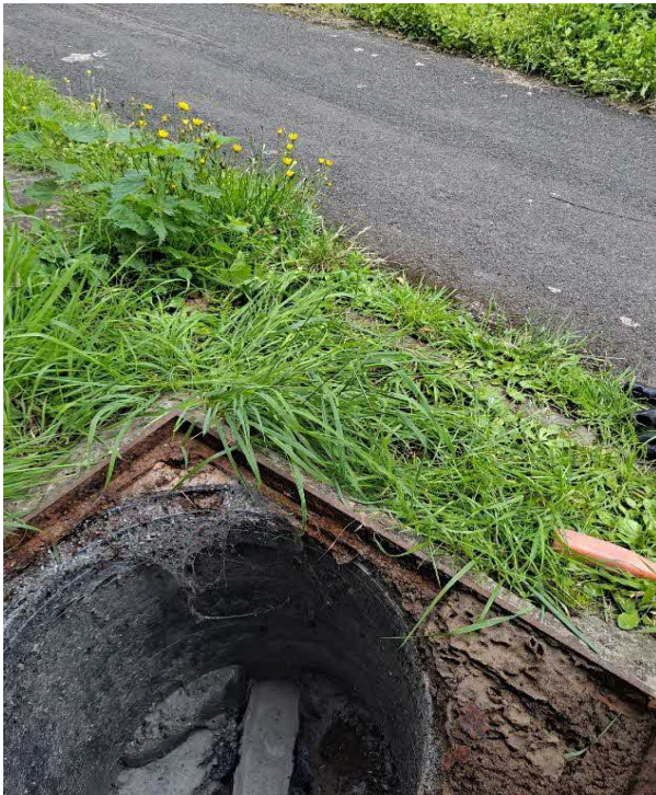
MH3 blocked downstream
