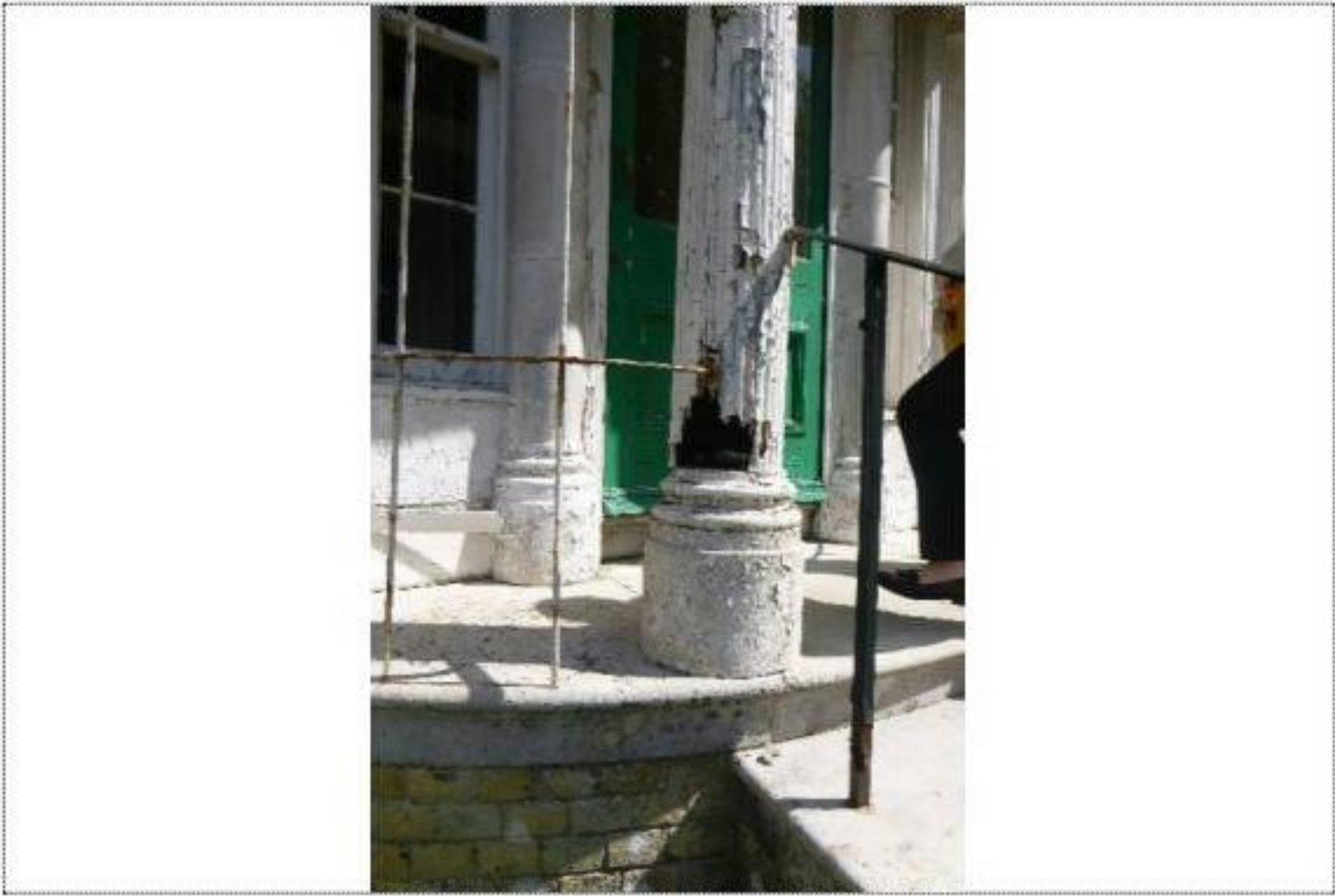
Photograph 9 - South Elevation Decayed Column
