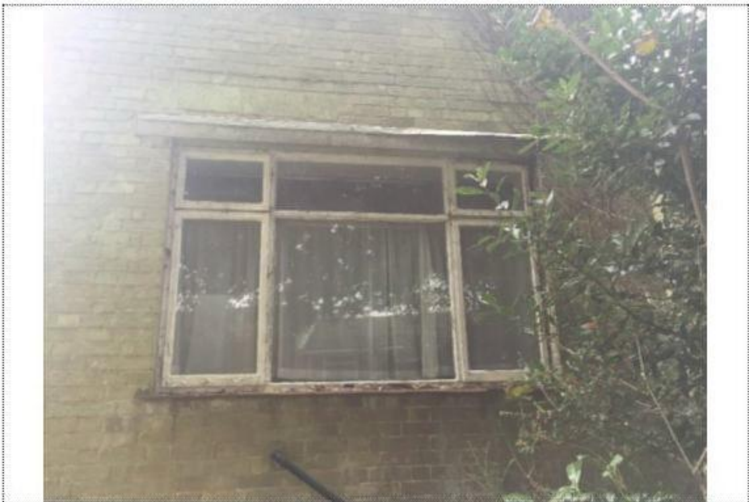
Photograph 20 - Single Storey Extension Kitchen Window and Exposed Lintel
