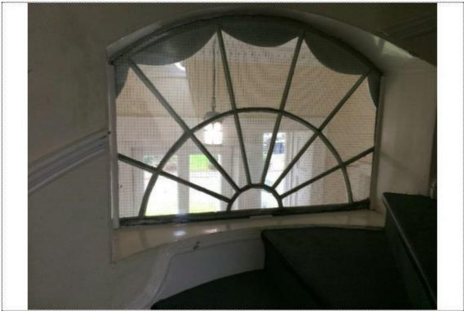
Photograph 29 – Georgian Wire Stairwell Glazing
