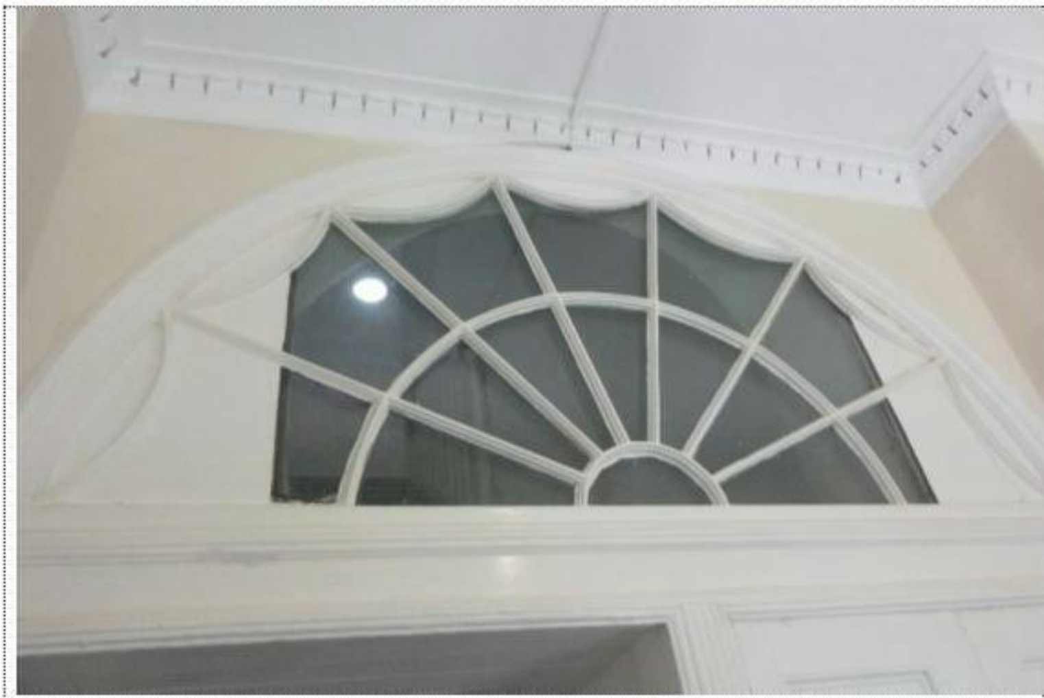
Photograph 30 – Georgian Wire Stairwell Glazing
