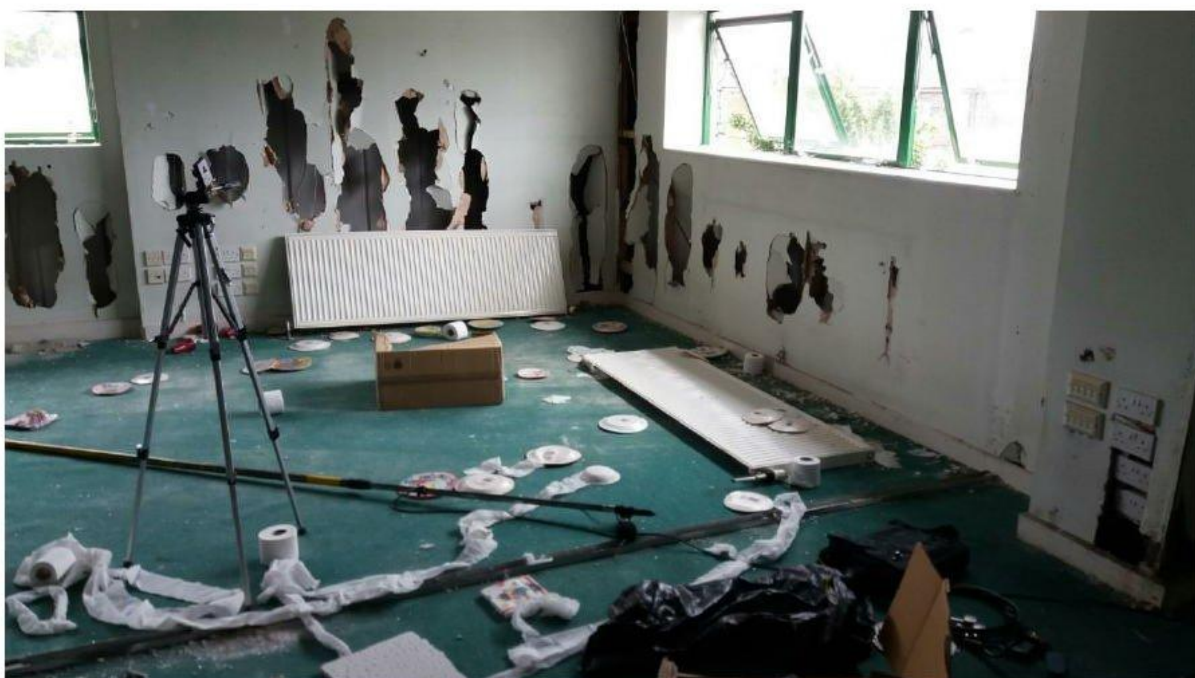
Photo 4 Equipment vandalised – the building had been vandalised earlier
