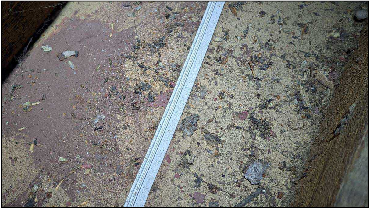
Photo 5 –Scattered bat droppings in the garage loft.
