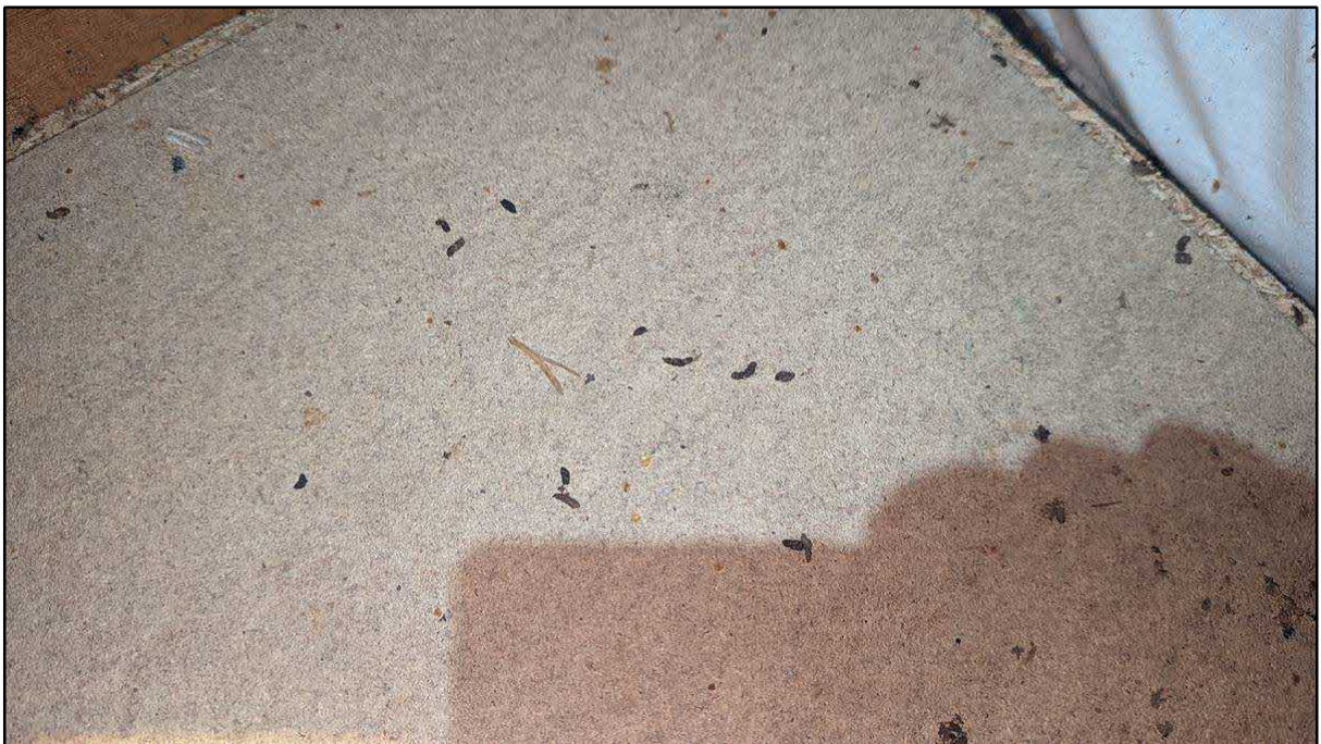
Photo 4 –Scattered bat droppings in the main loft.
