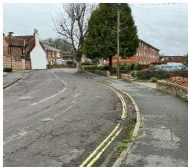
Photograph 16: Grove Road Conditions
