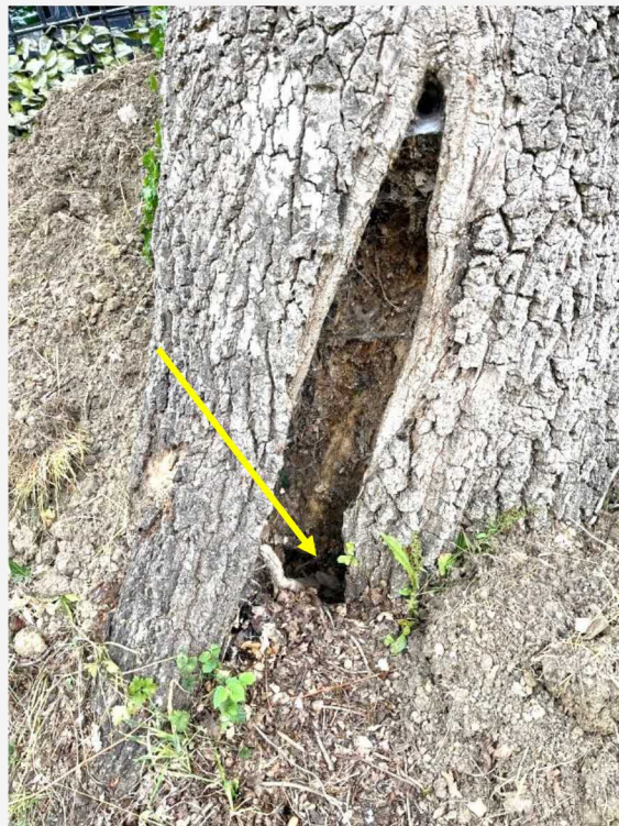
T1 Extensive basal cavity to Northwest side.
