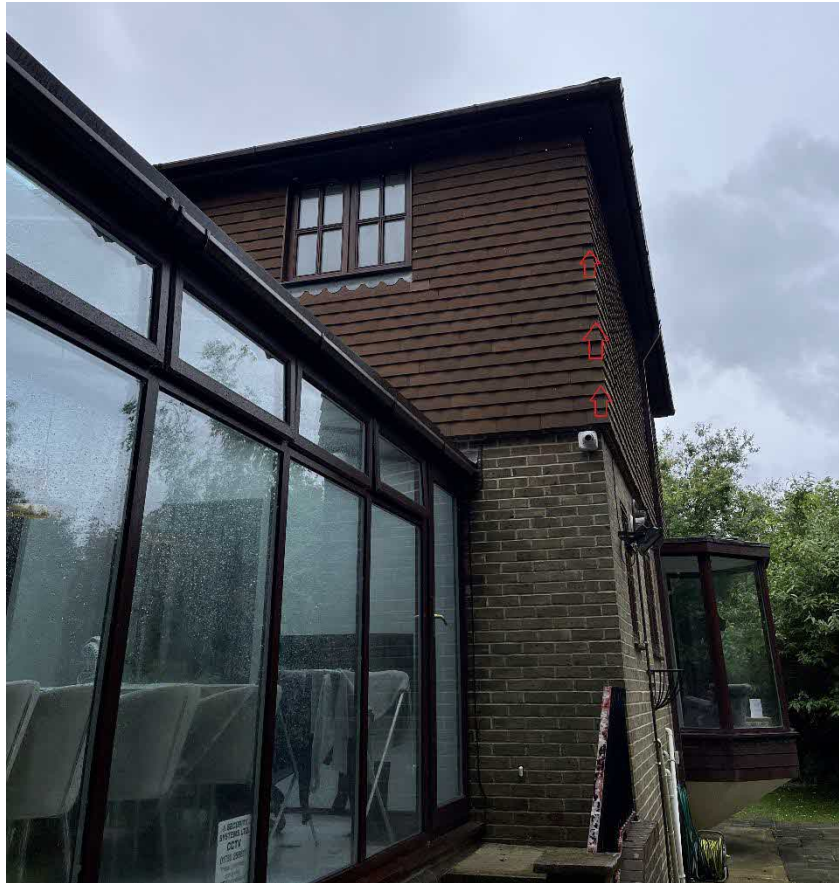
Figure 8. Northern and eastern elevations looking west: Red arrows indicate potential openings into under-tiles spaces.
