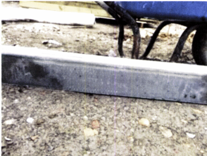
Standard Concrete Edgings
