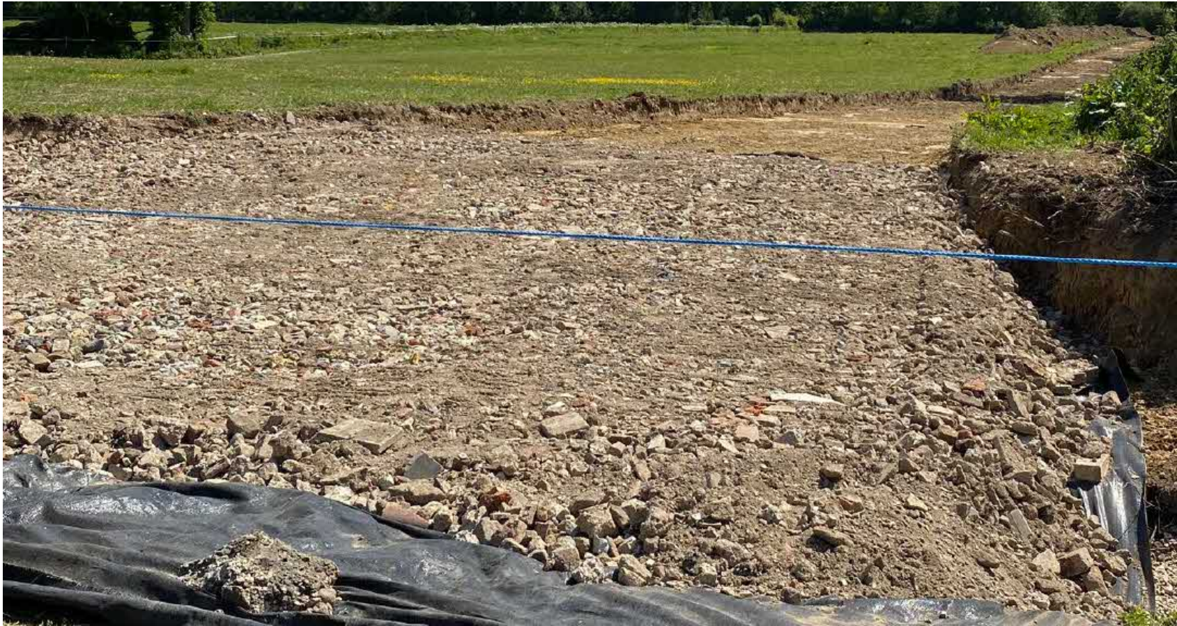
Road subbase laid on geotextile. Note presence of non uniform site material, clearly not properly graded, also clat pipes, bricks and other waste material which could degrade. Also note high level of fine material meaning road unlikely to be permeable
