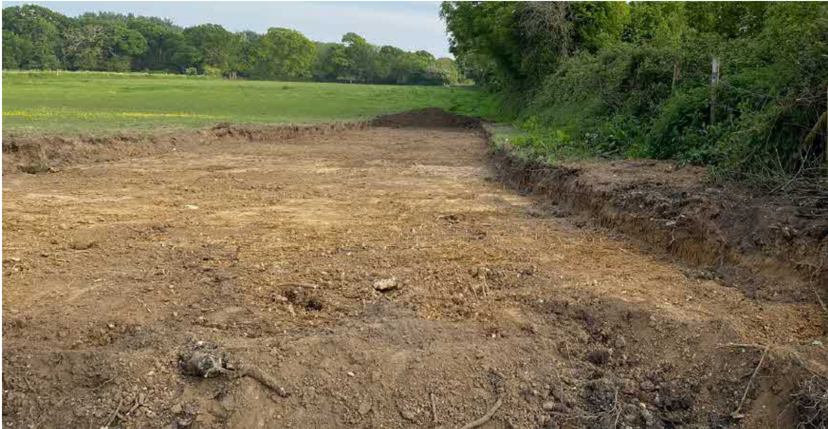
Reduced level dig for new road, no CBR testing appears to have been carried out to enable road design
