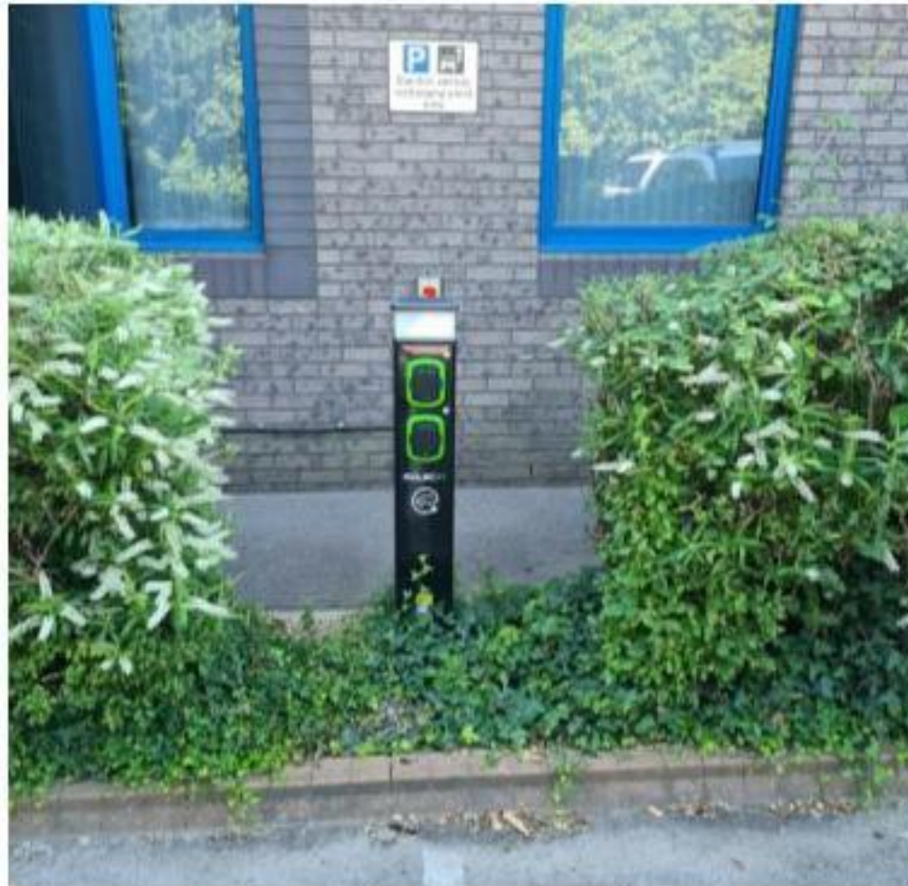
Photograph 10: Existing Electric Vehicle Charging Point
