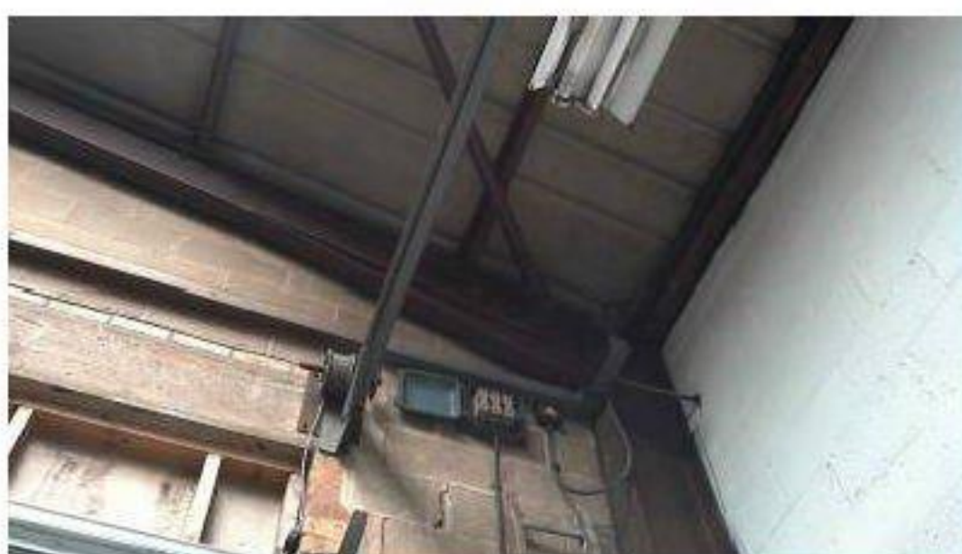
Ref. Sample 11: Workshop Building. Ground Floor. Bay 3. Woven flash pads within high level fuse box north west corner
