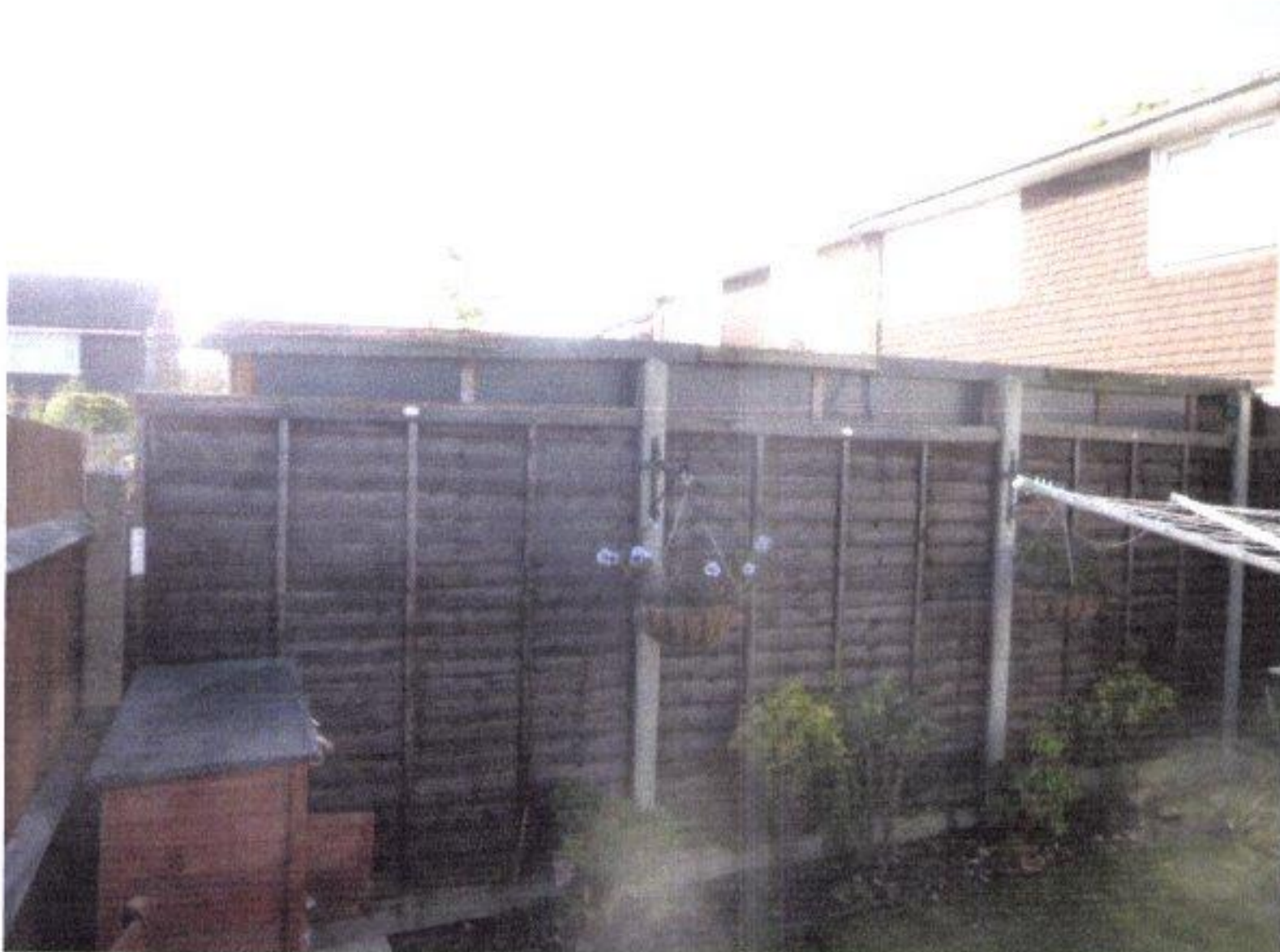
Picture 1) View from our rear garden to number 29, all that can be seen is black plastic cladding and mouldy wood.
