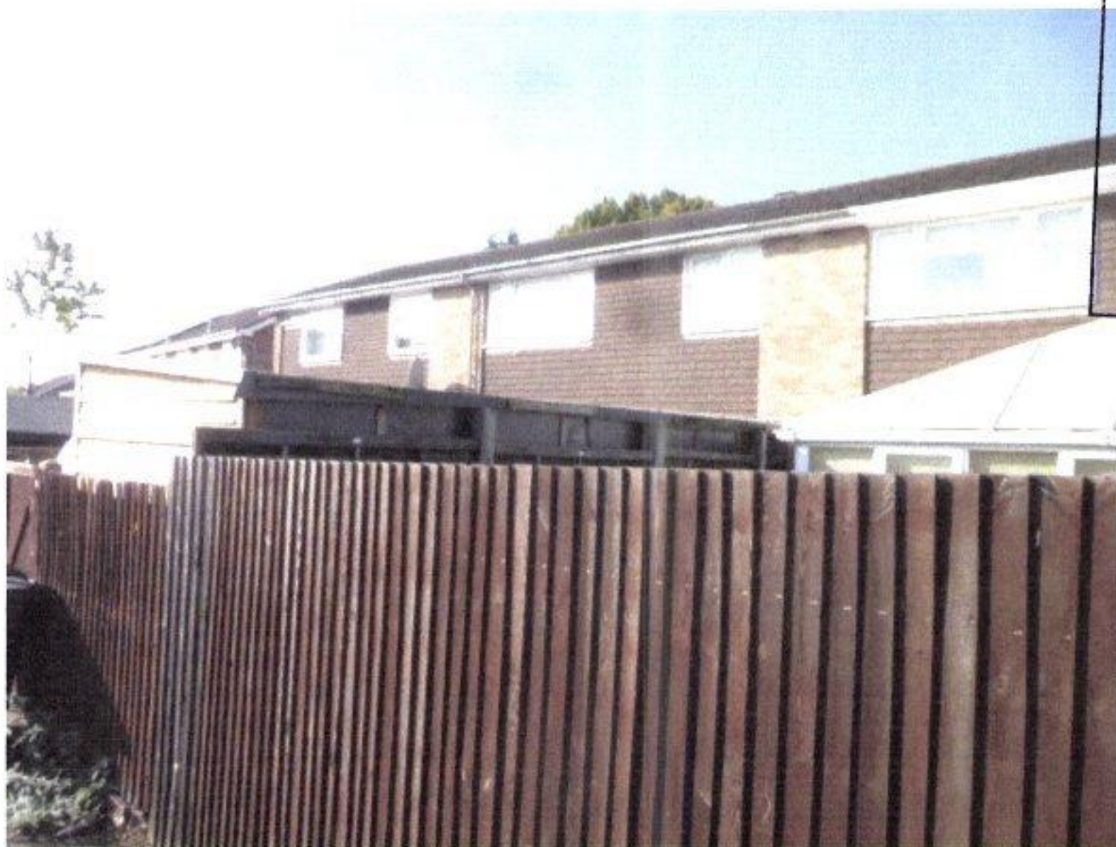
Picture 2) View from the rear car park. Again black plastic cladding and mouldy wood.
