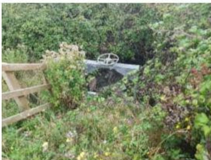
Photo 11: Manual flood gate valve
