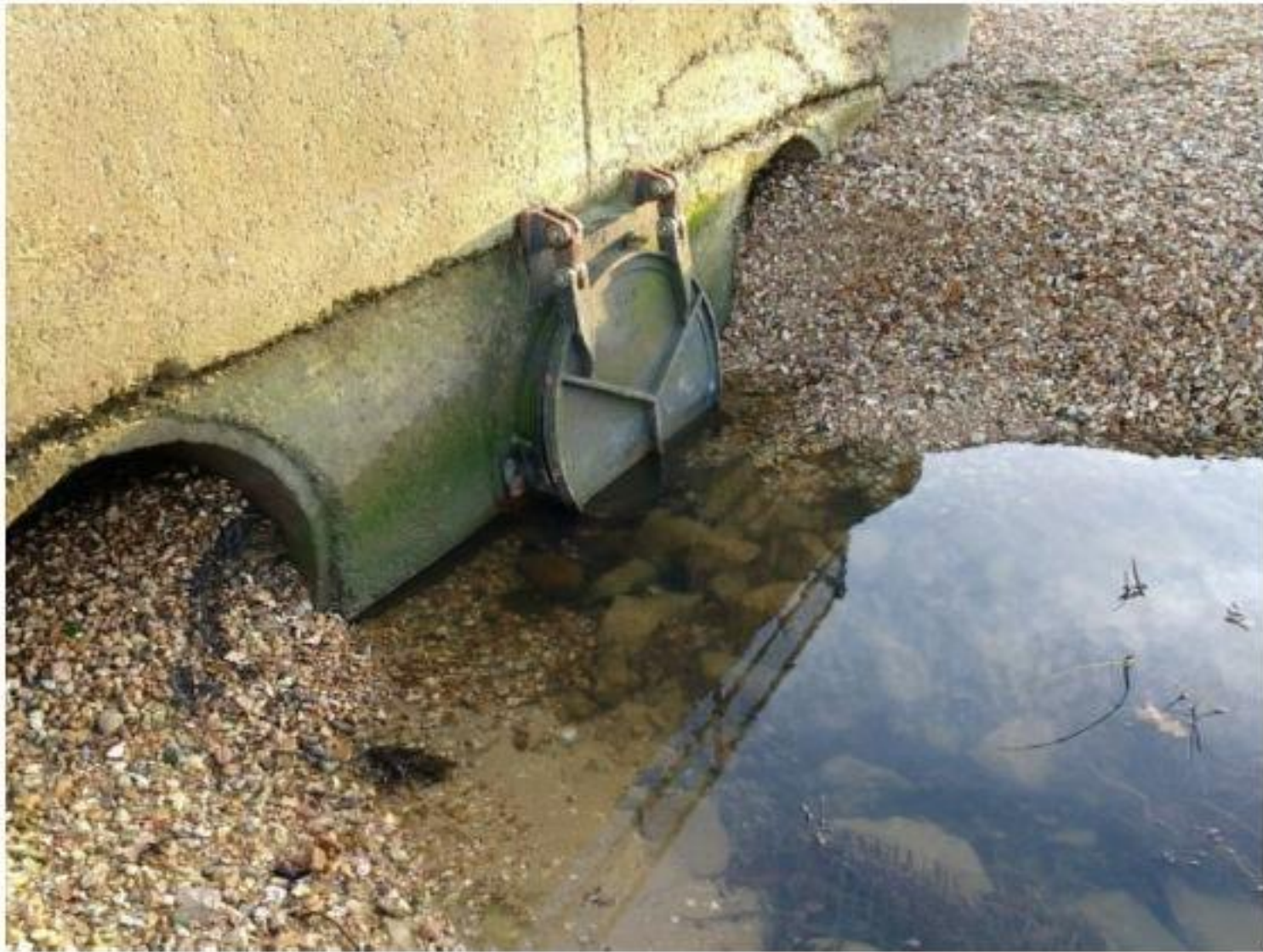
November 2017 - Shingle blocking drainage channel west side of Hayling Island
