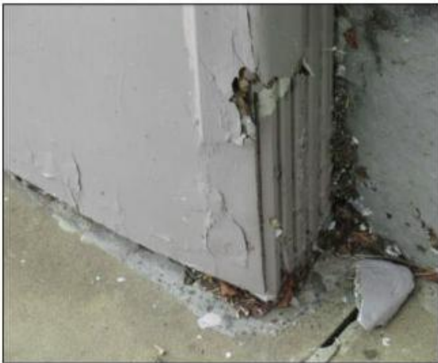
Woodwork rotten Will require repairing
