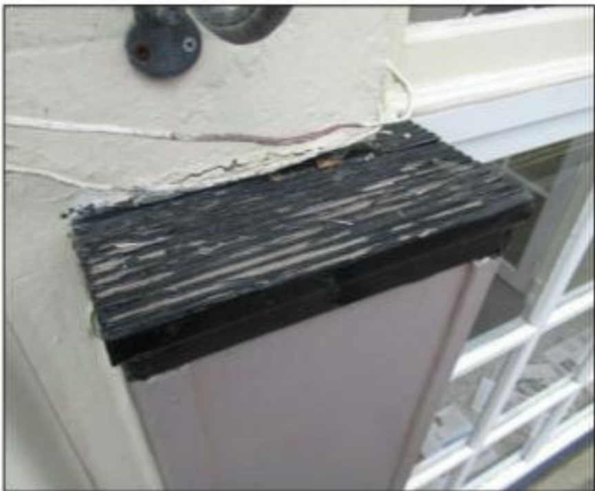
Top columns are peeling Will require repainting
