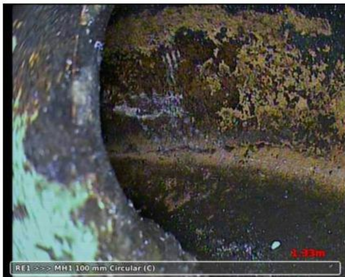
20191010-084757-snap0004.jpg, 00:01:15, 1.33 m Line deviates left
