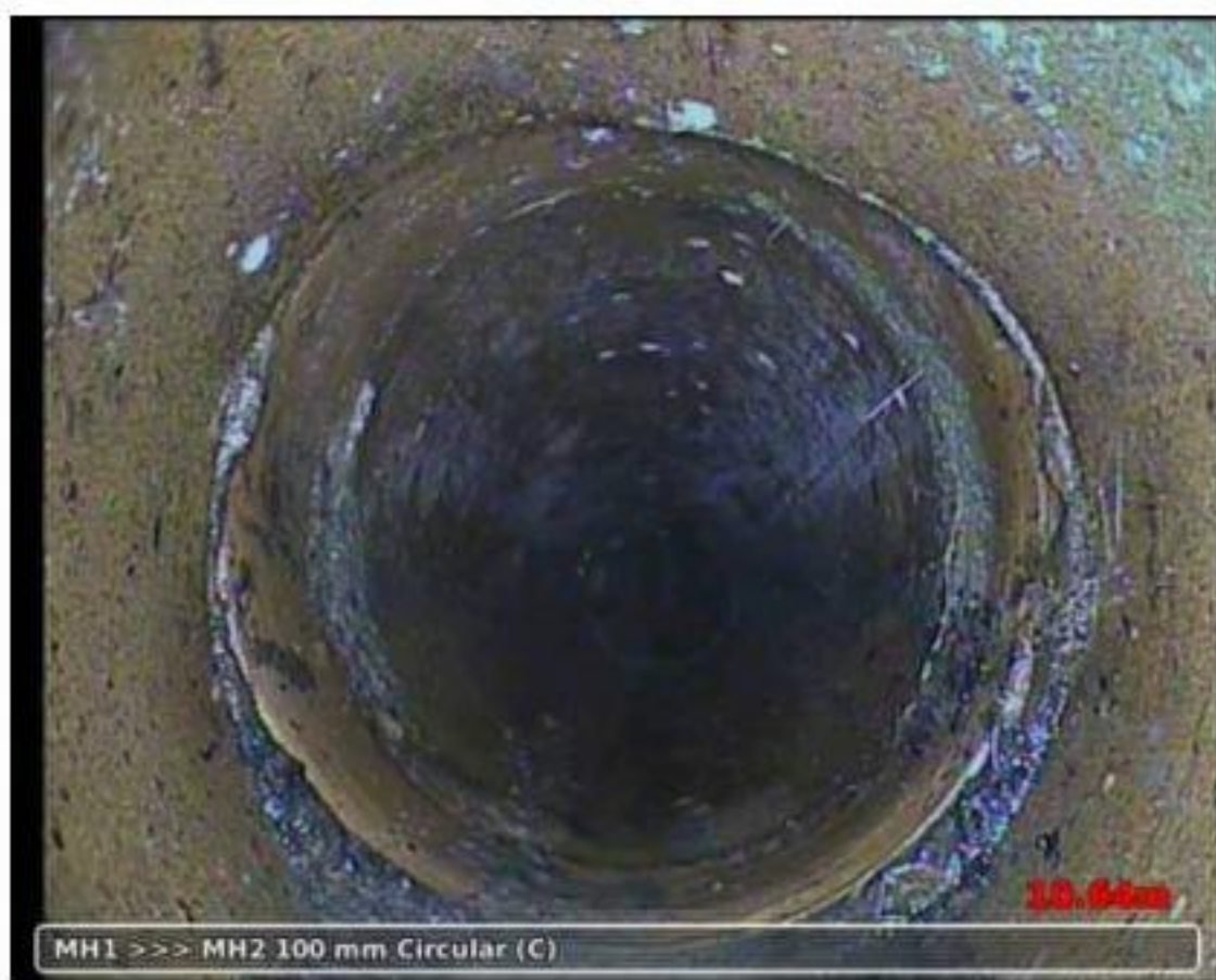
20191010-090906-snap0010.jpg, 00:03:32, 10.64 m Crack, circumferential, from 12 to 12 o'clock
