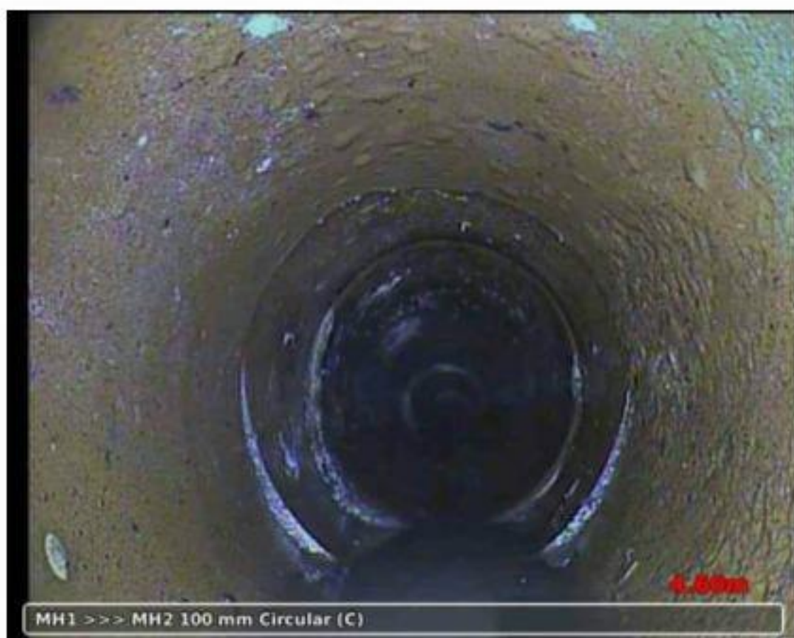
20191010-090906-snap0005.jpg, 00:01:42, 4.60 m Crack, circumferential, from 12 to 12 o'clock
