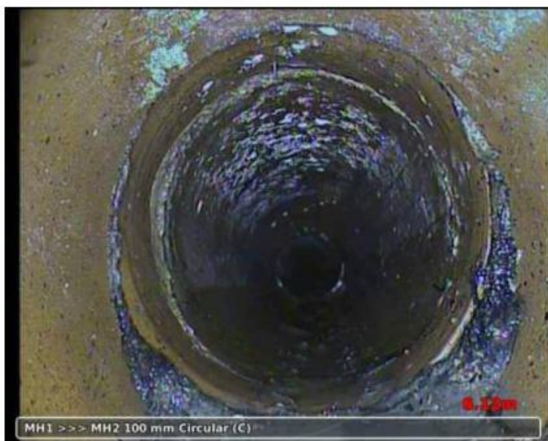
20191010-090906-snap0007.jpg, 00:02:24, 6.12 m Crack, circumferential, from 12 to 12 o'clock
