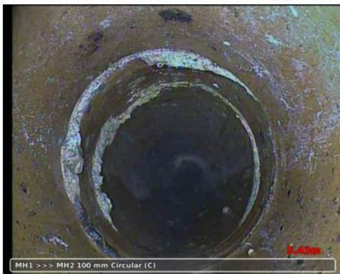
20191010-090906-snap0006.jpg, 00:02:01, 5.43 m Crack, circumferential, from 12 to 12 o'clock
