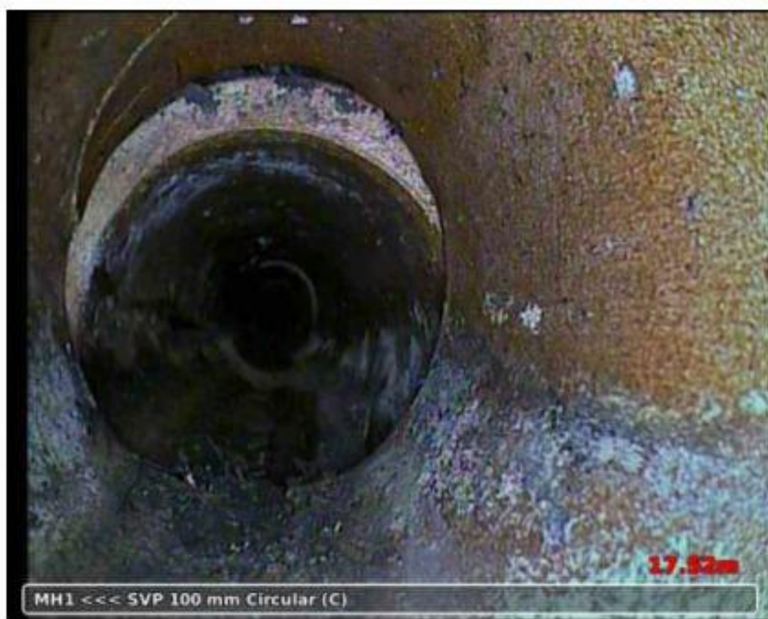
20191010-085806-snap0008.jpg, 00:04:25, 17.52 m Joint displaced, 10 mm displacement
