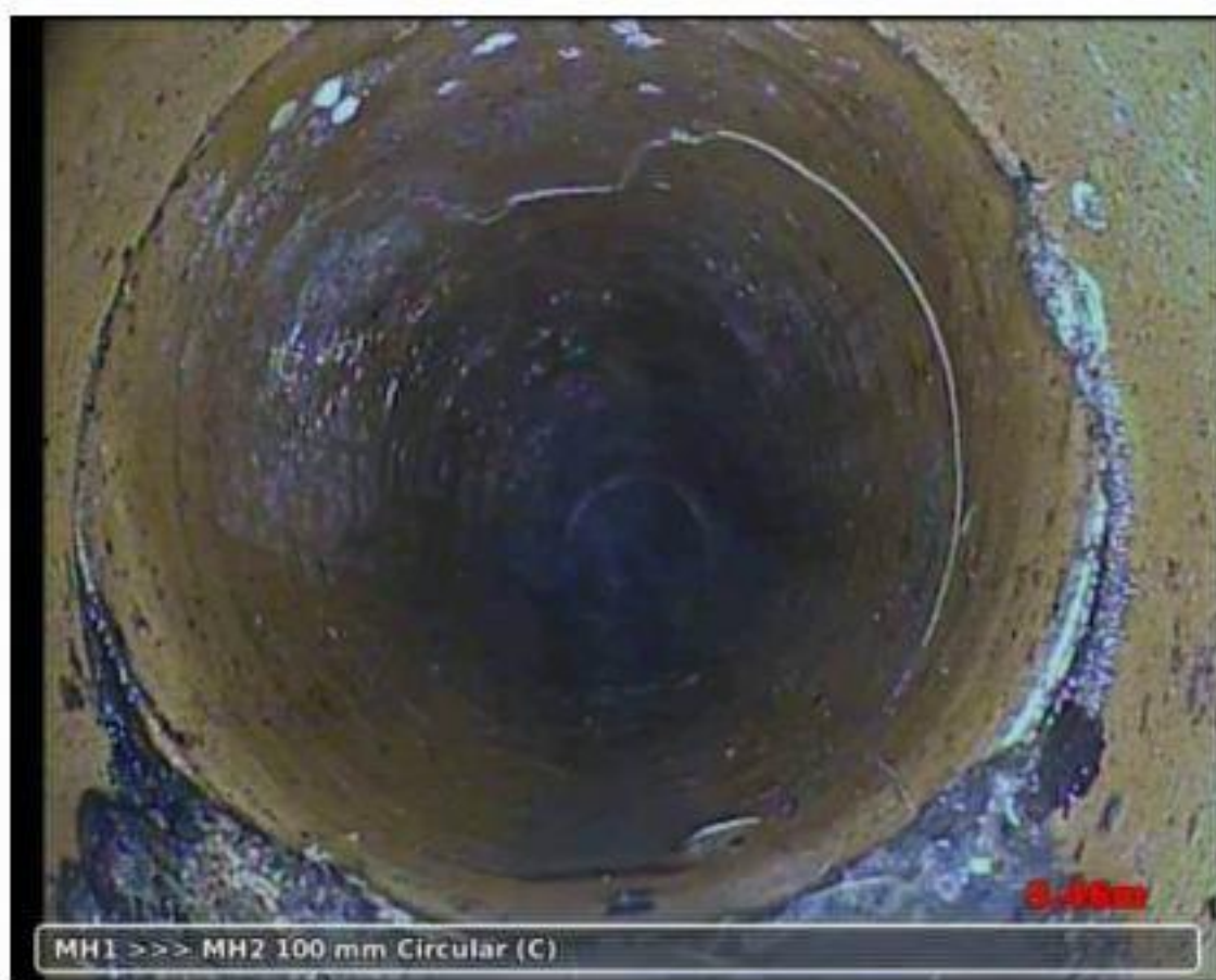
20191010-090906-snap0004.jpg, 00:01:19, 3.46 m Crack, circumferential, from 12 to 06 o'clock
