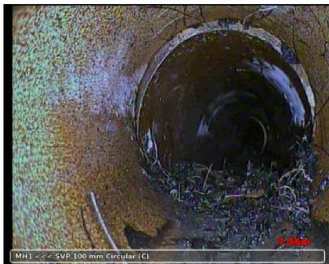
20191010-085806-snap0003.jpg, 00:01:29, 7.56 m Roots, mass, 10 % cross-sectional area loss
