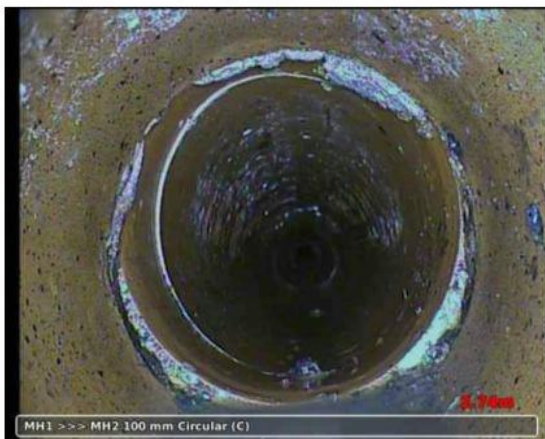
20191010-090906-snap0003.jpg, 00:00:47, 2.70 m Crack, circumferential, from 06 to 12 o'clock
