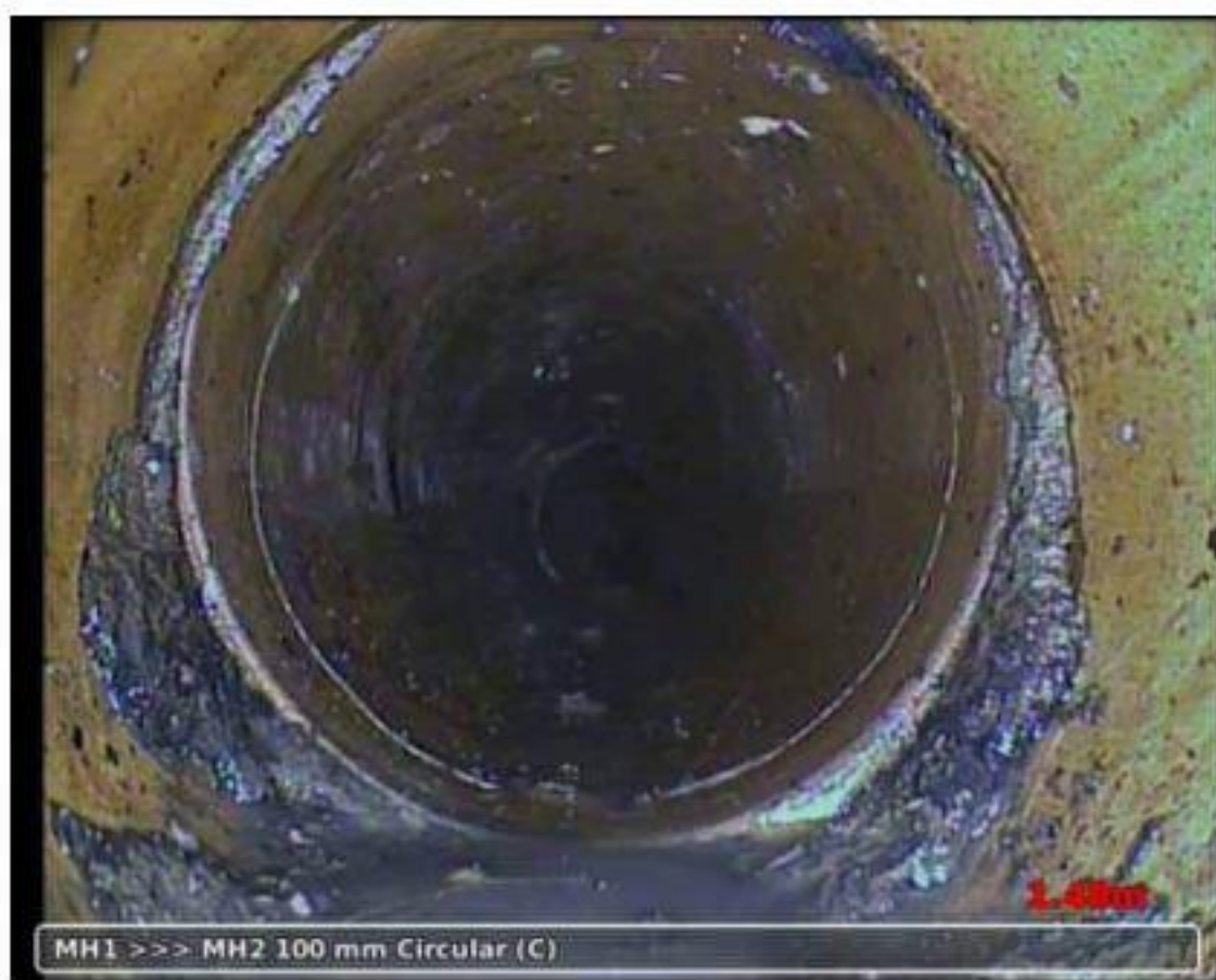
20191010-090906-snap0002.jpg, 00:00:26, 1.48 m Crack, circumferential, from 03 to 10 o'clock
