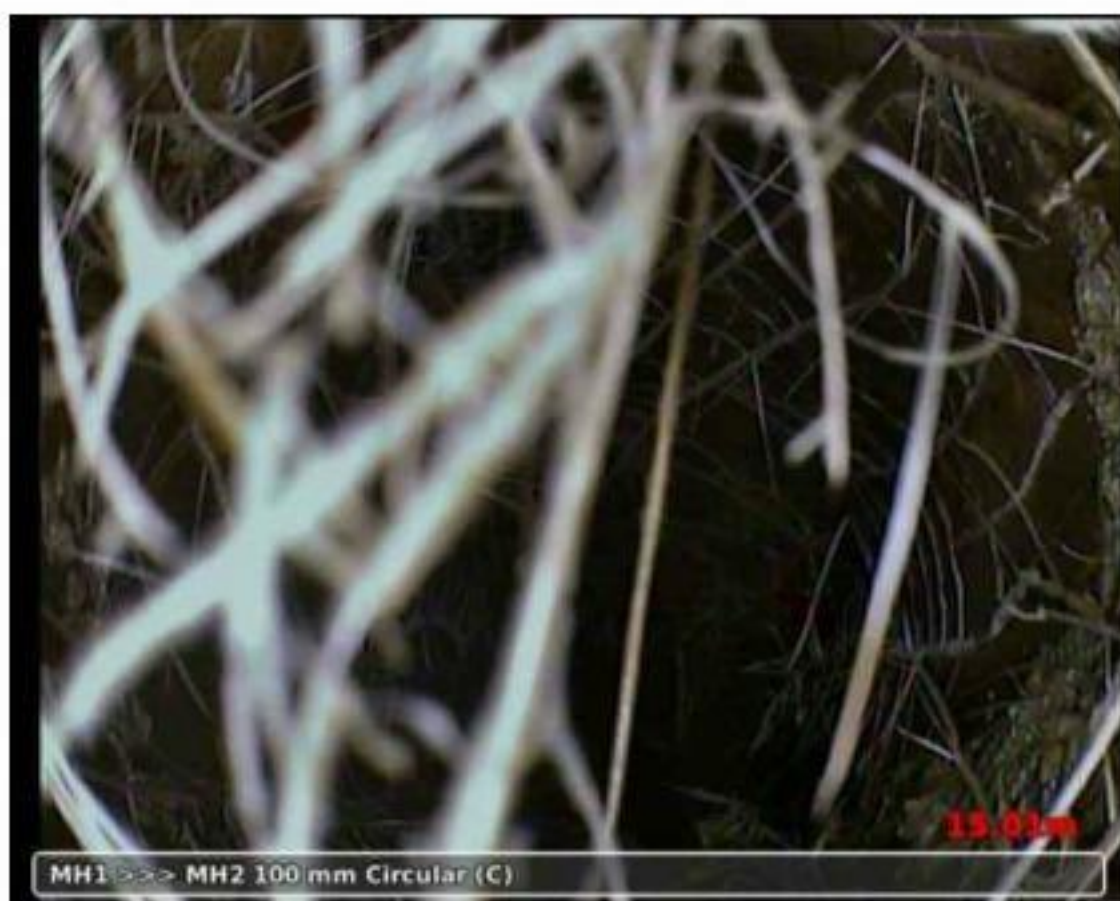
20191010-090906-snap0015.jpg, 00:05:03, 15.01 m Roots, mass, 40 % cross-sectional area loss
