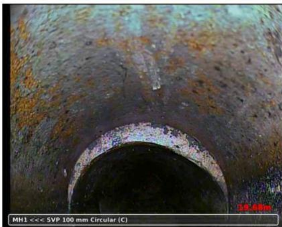
20191010-085806-snap0010.jpg, 00:05:58, 19.68 m Joint displaced, 10 mm displacement
