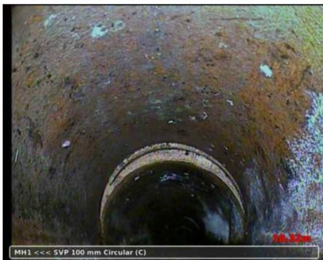
20191010-085806-snap0009.jpg, 00:05:11, 18.32 m Joint displaced, 10 mm displacement
