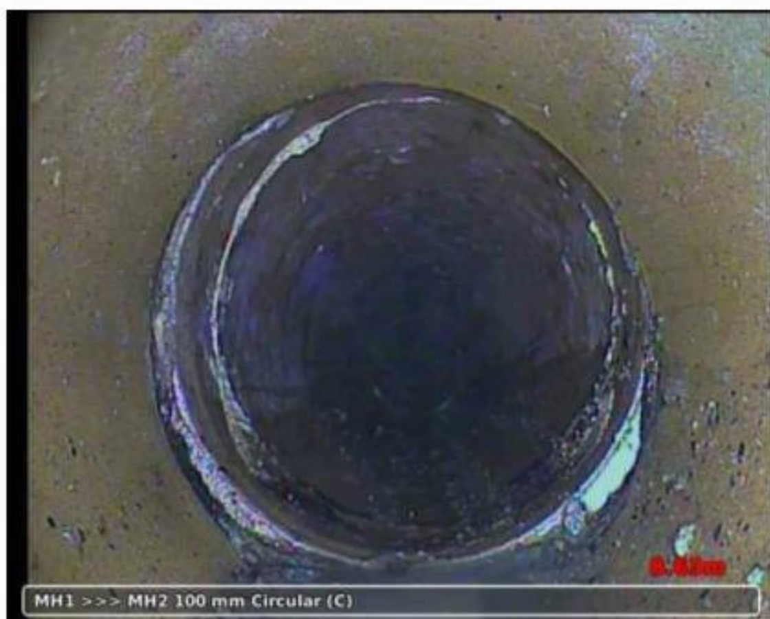
20191010-090906-snap0009.jpg, 00:03:05, 8.63 m Crack, circumferential, from 12 to 12 o'clock
