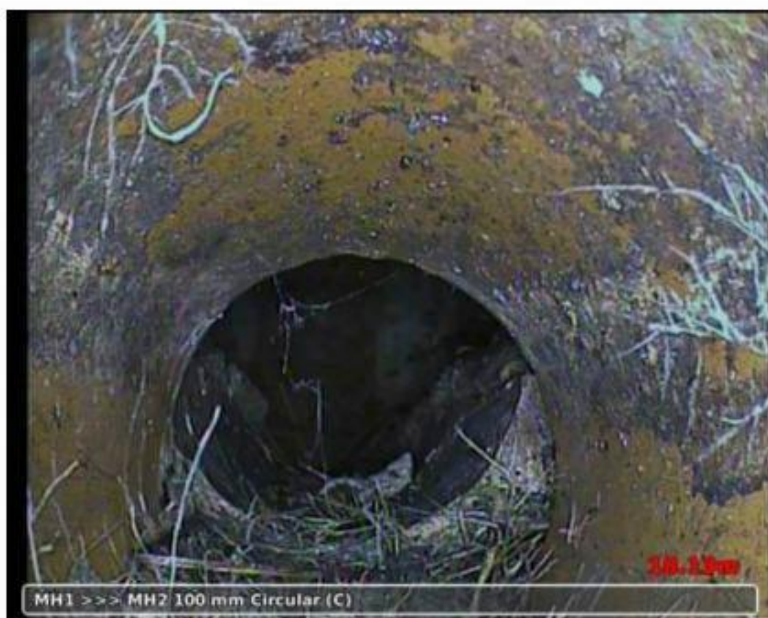
20191010-090906-snap0017.jpg, 00:05:52, 18.09 m Joint displaced, 20 mm displacement
