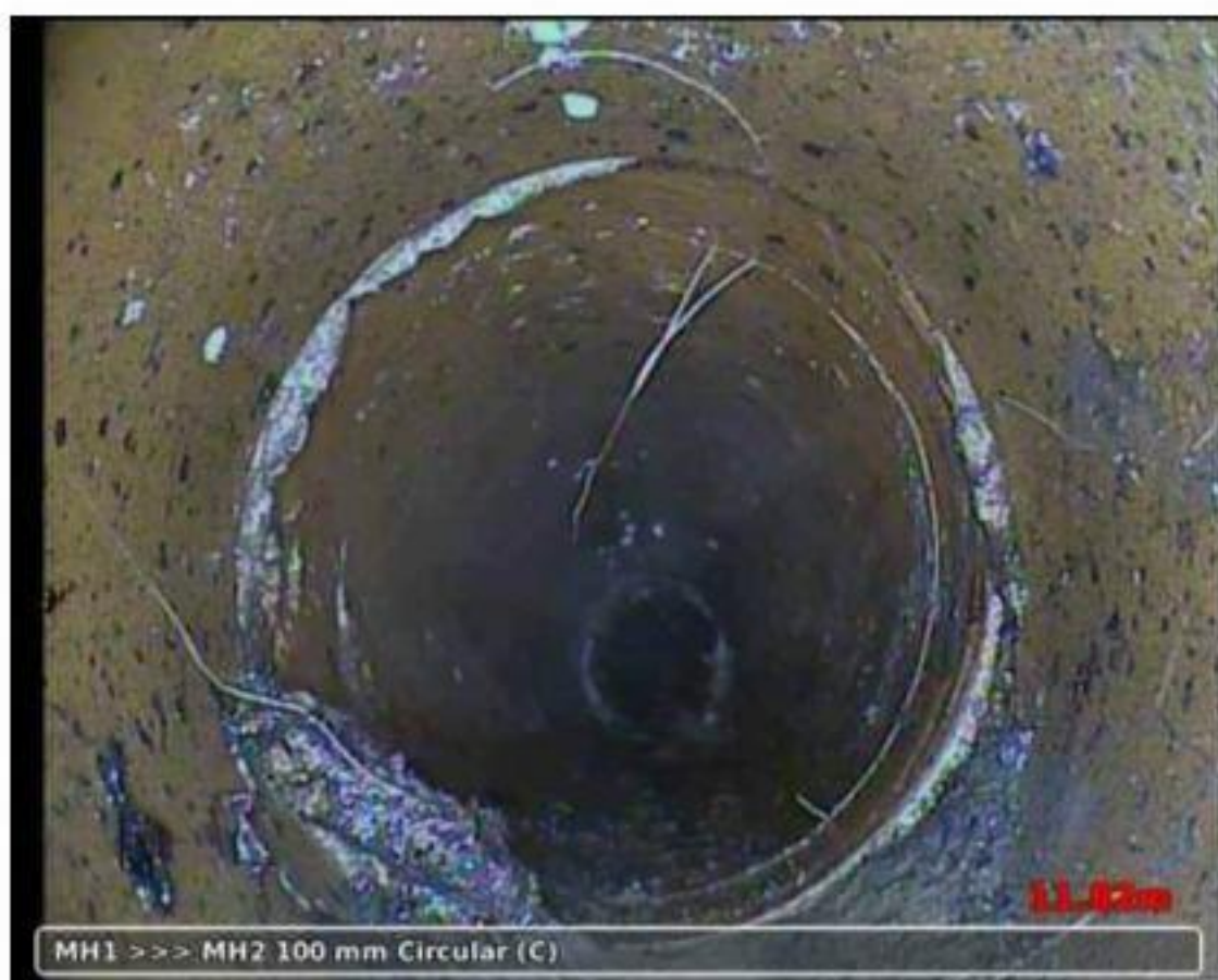
20191010-090906-snap0011.jpg, 00:03:56, 11.82 m Crack, circumferential, from 12 to 12 o'clock
