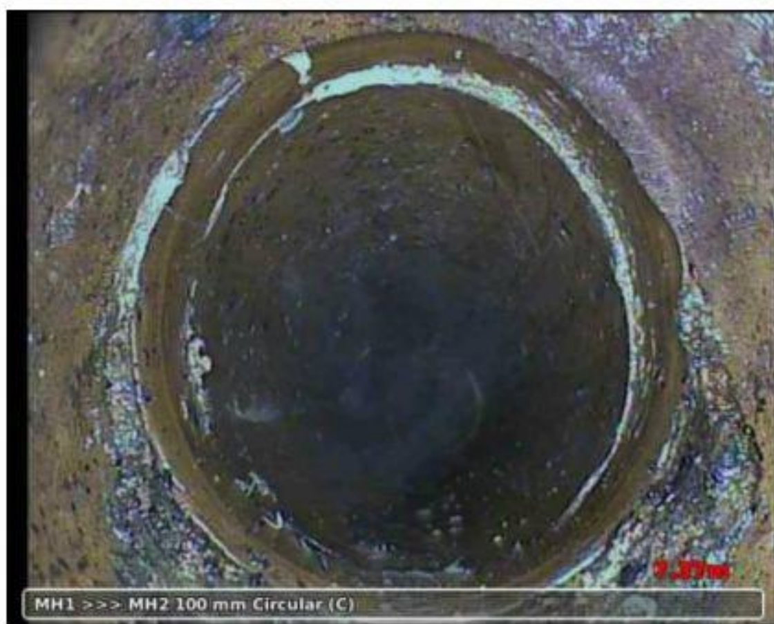
20191010-090906-snap0008.jpg, 00:02:44, 7.37 m Crack, circumferential, from 12 to 12 o'clock
