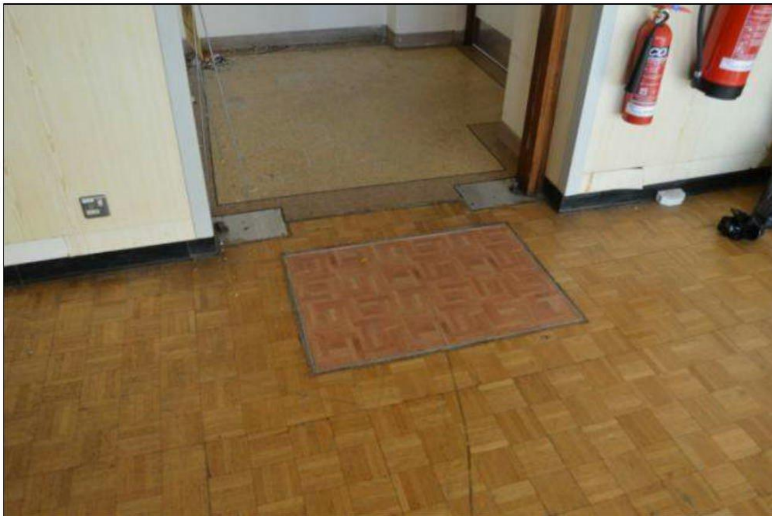
Photograph twelve: underfloor services in the Colt office block, looking northeast.
