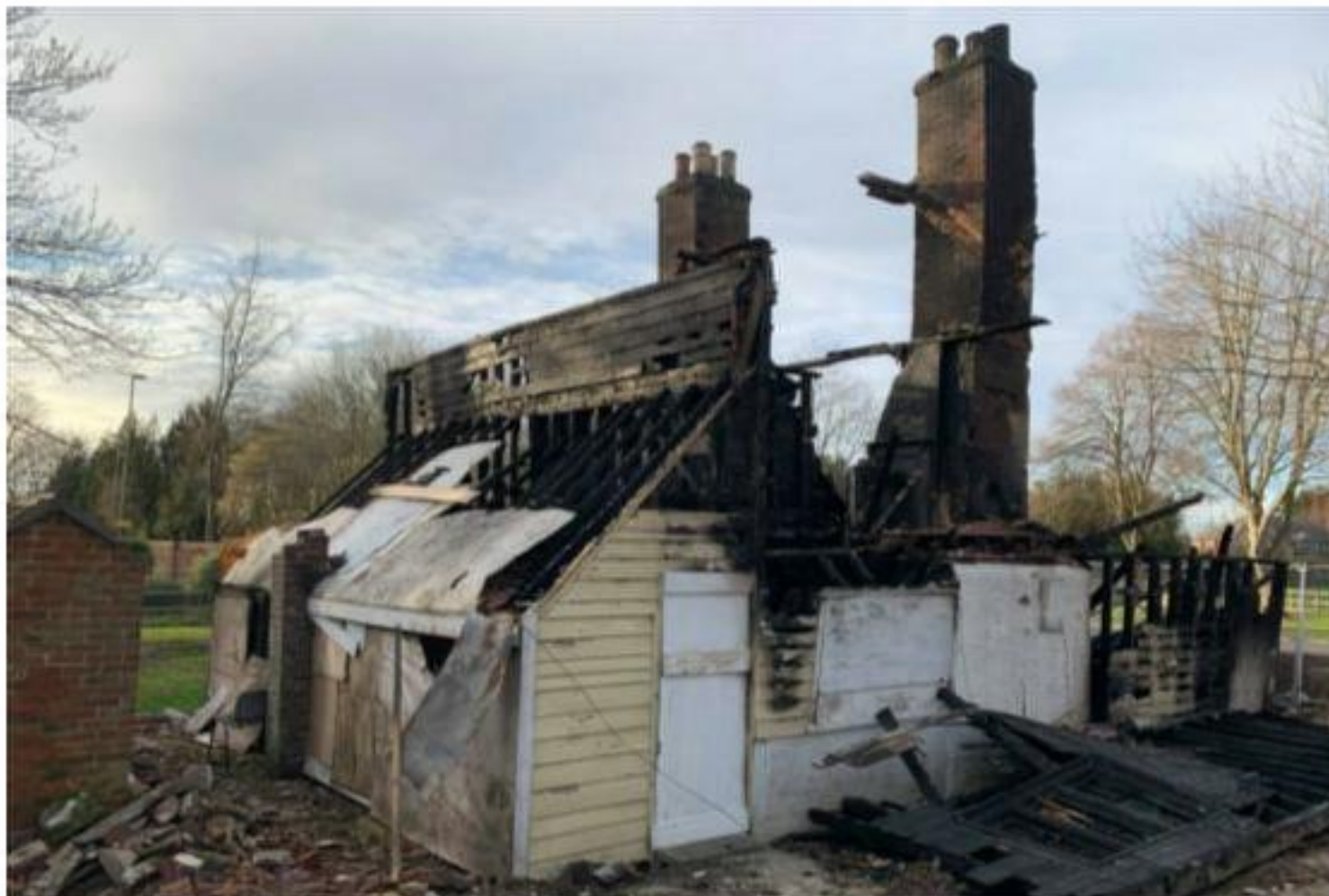
Figure 3: Post-Fire Damage (Jan 2019)
