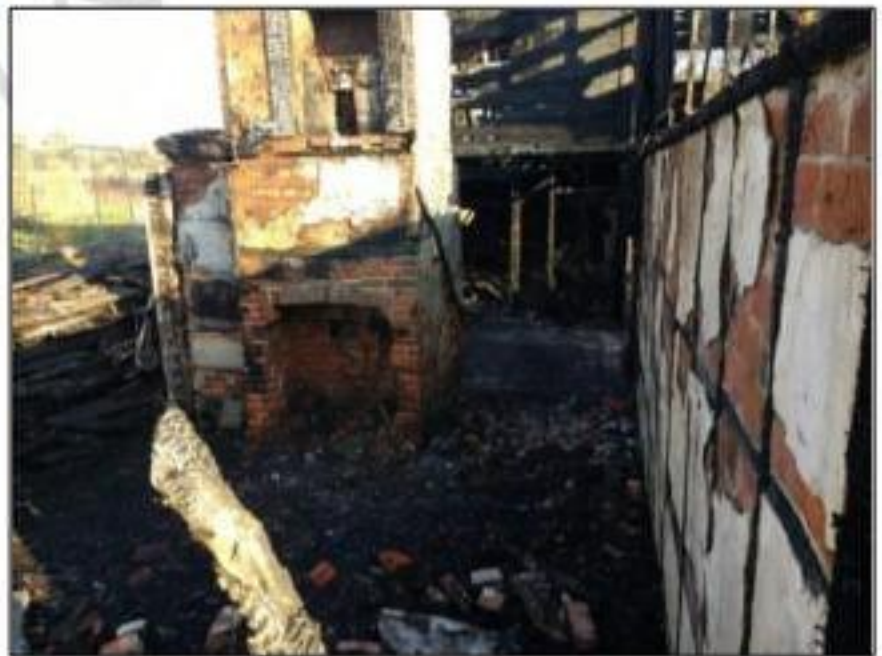
Figure 24: The cottages after the devastating fire (Jan, 2019)
