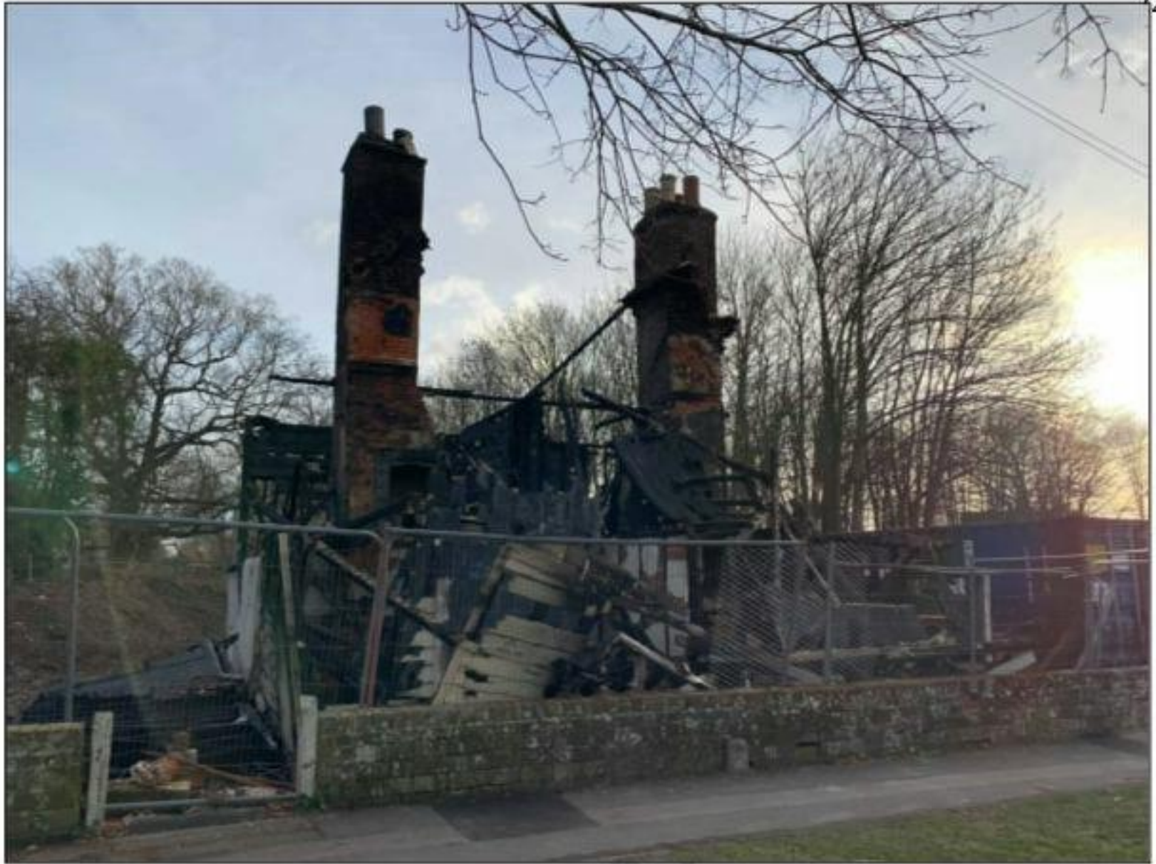
Figure 22: The cottages after the devastating fire (Jan, 2019)
