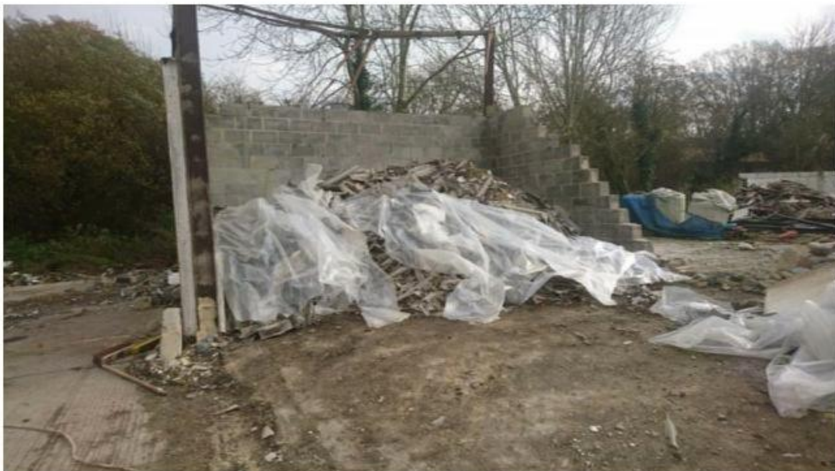
Plate 3 View of partially covered stockpiled demolition waste including possible ACM's
