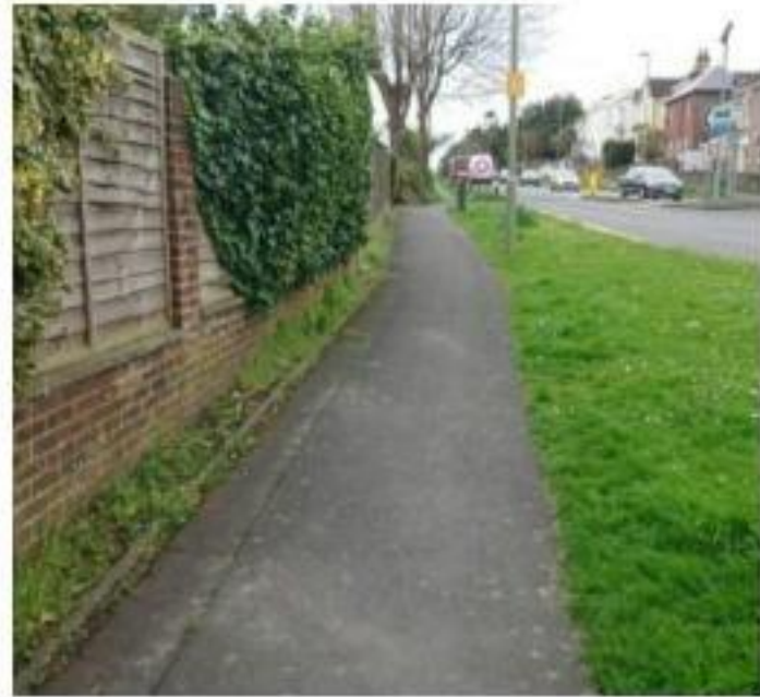
Photograph 49: Footway Conditions along Bedhampton Road
