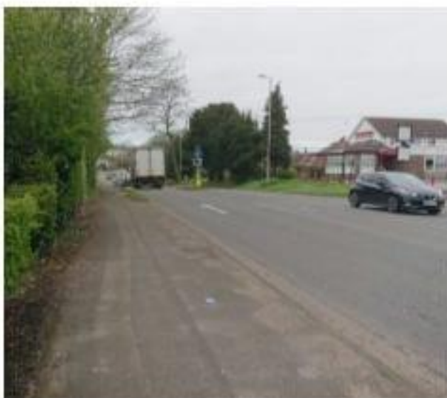
Photograph 46: Footway Conditions along Bedhampton Road
