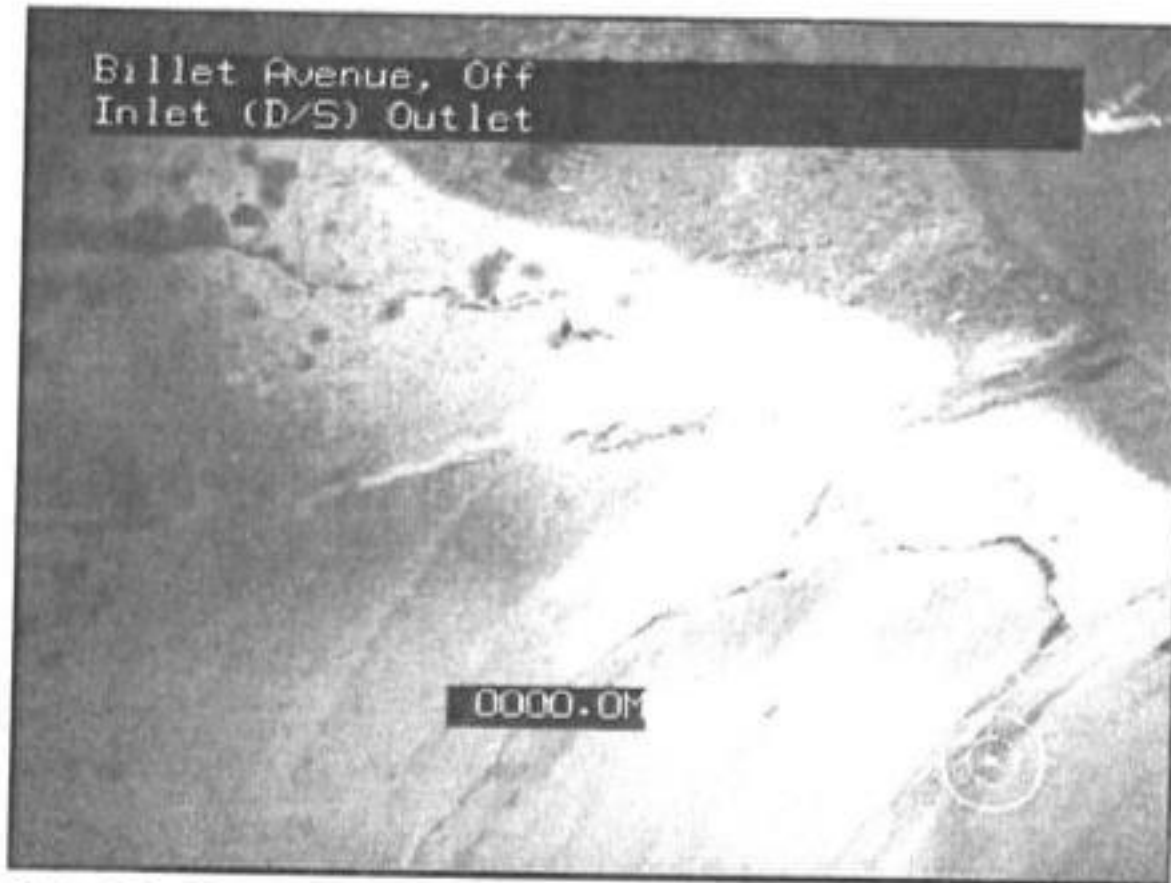
Photo: 6_6a, Tape No.: 1, 00:00:00 0m, Longitudinal Fracture at 05 o'clock
