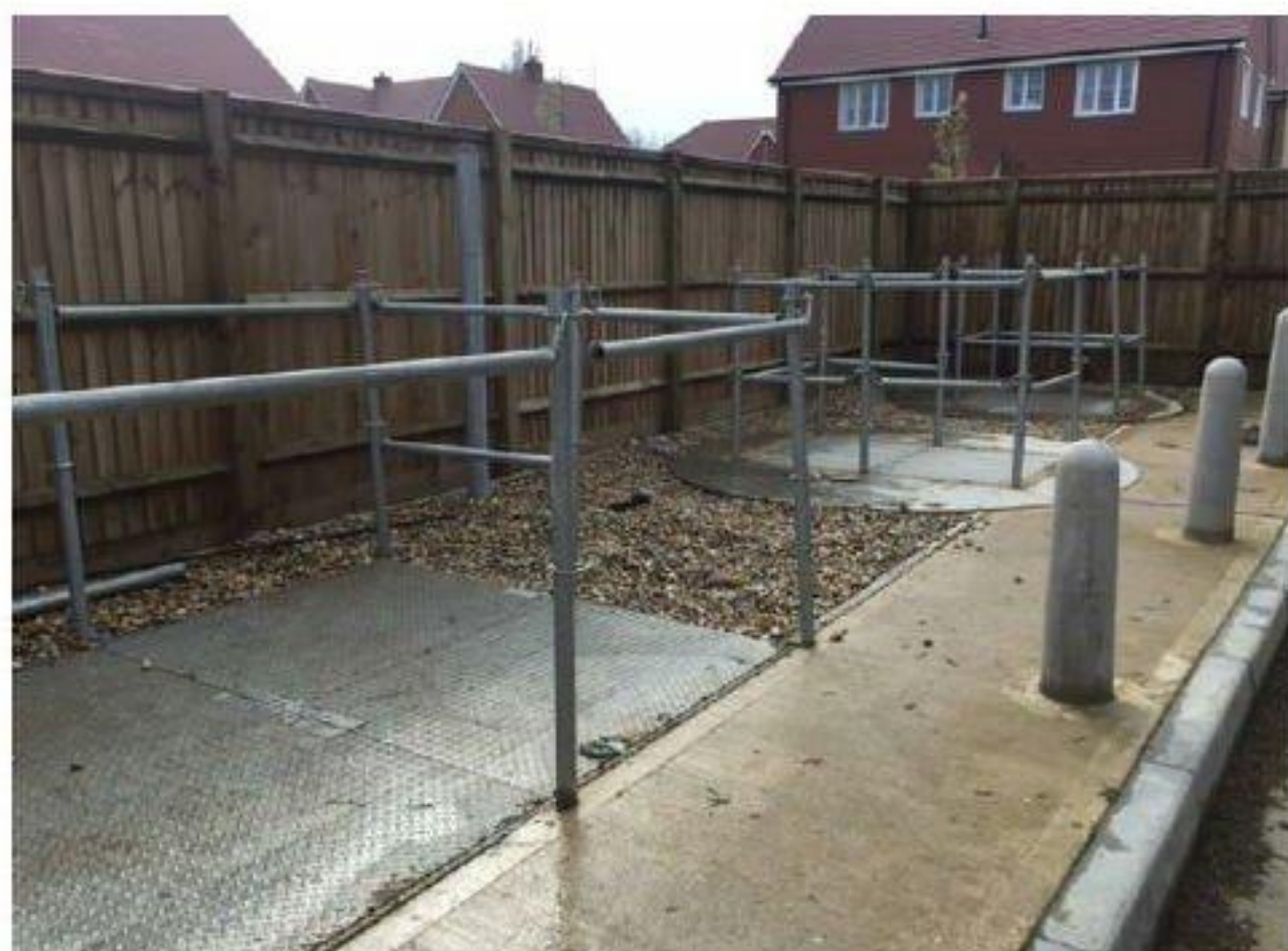
Pumping station (covers closed)
