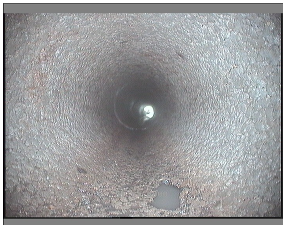
Photo: 1_1_12_A.JPG 40.88m, Hole in drain/sewer, from 5 to 6 o'clock
