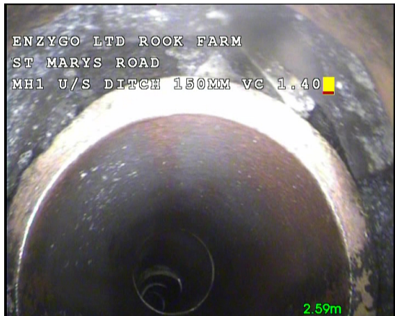
Photo: 3_3_16_A.jpg 2.59m, Joint displaced, large
